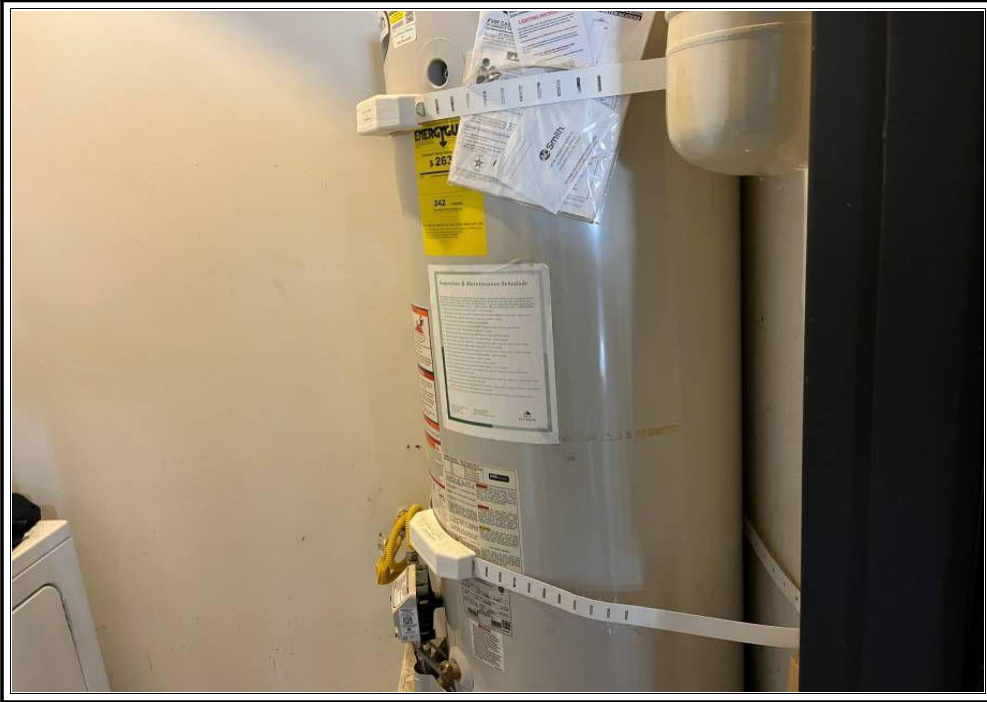
Interior Photo Garage Water Heater
