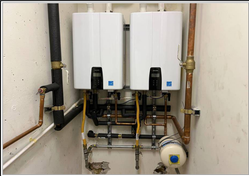
Interior Photo Tankless Water Heaters
