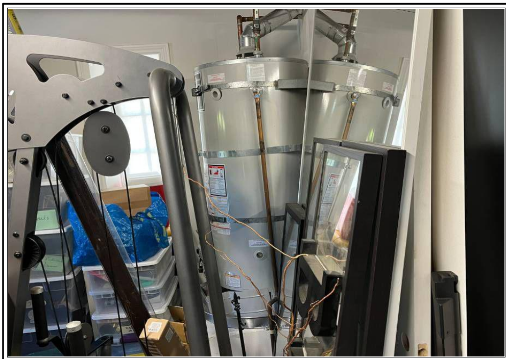
Interior Photo Water Heater
