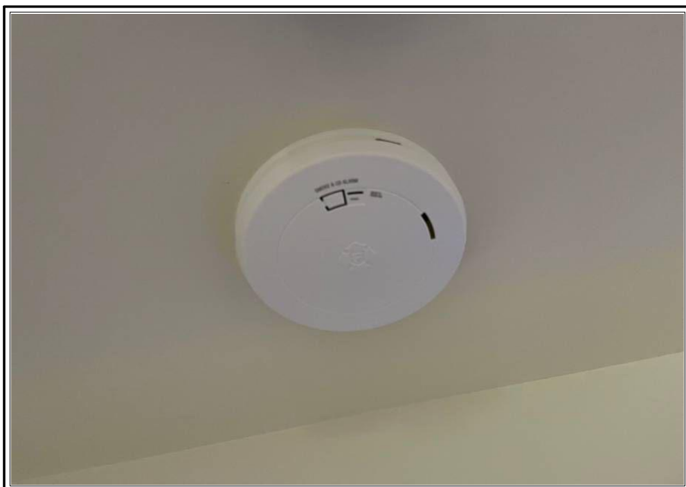
Interior Photo Smoke/CO Alarm
