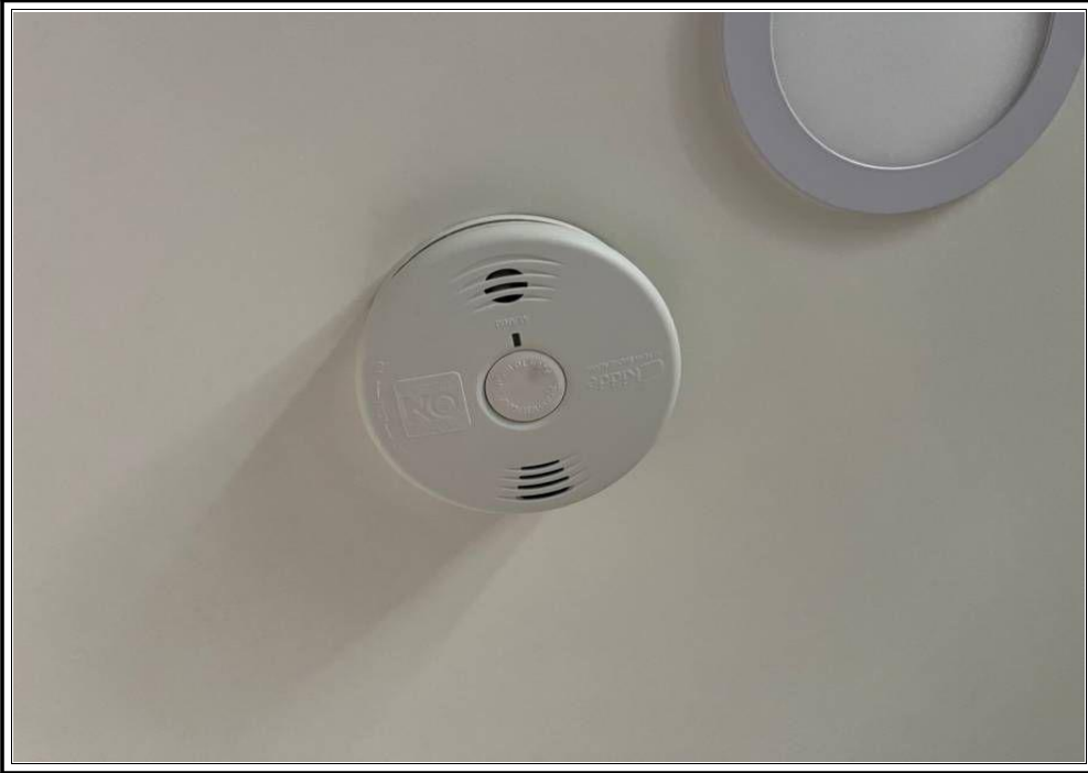
Interior Photo Smoke/CO Alarm
