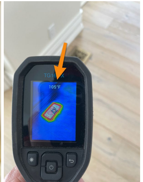
Example Noted At Dining Room
