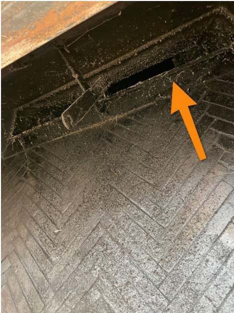
Example Noted At Dining Room
