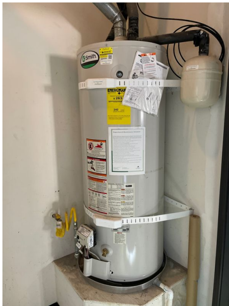
Example Noted At Garage
