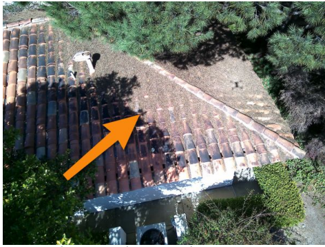
Example Noted At Pool House
