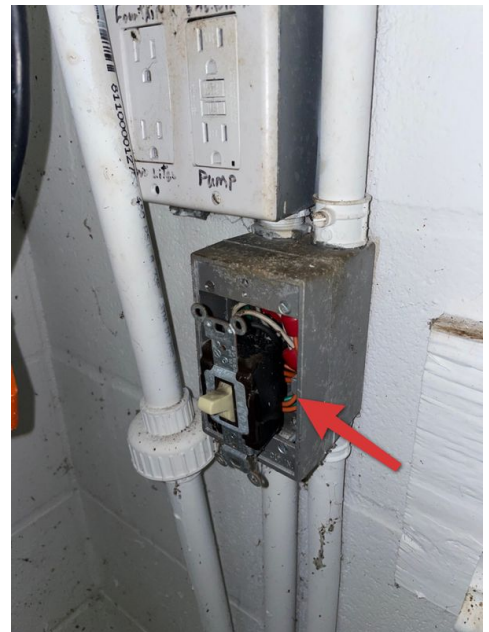
Example Noted At Pool Equipment Room
