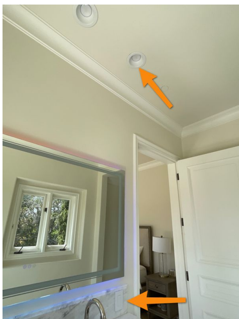
Example Noted At Bedroom 4 Bathroom
