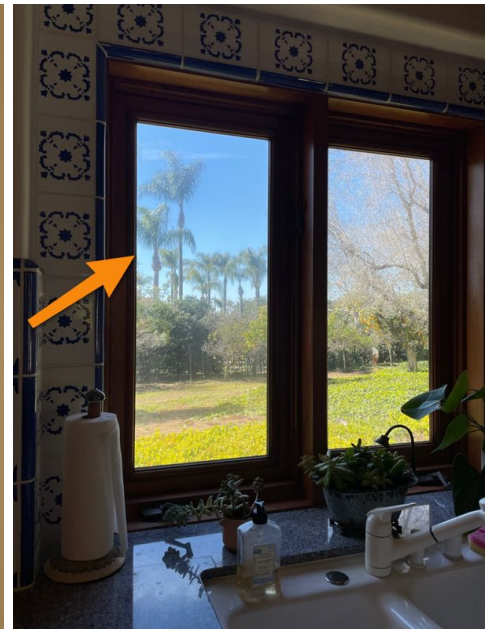
Example Noted At Pool House Kitchen
