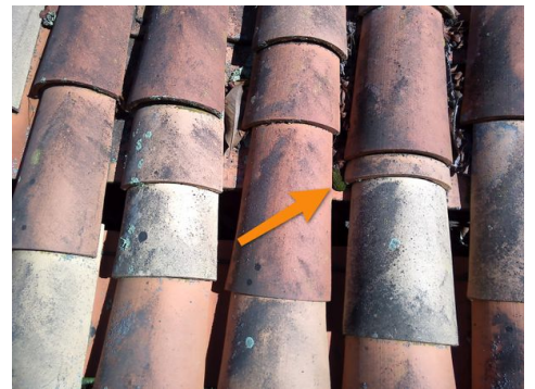
Example Noted At Roof
