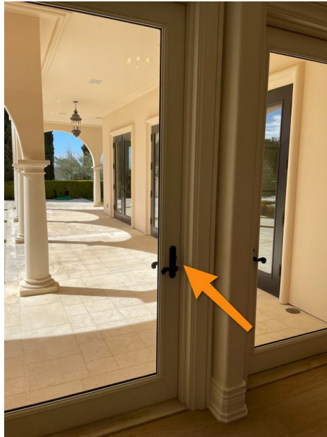
Example Noted At Hallway
