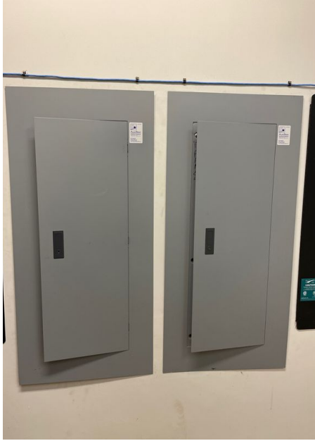
Example Noted At Basement
