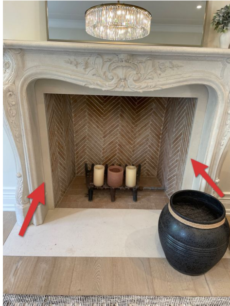
Example Noted At Living Room
