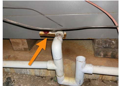
Example Noted At Crawlspace
