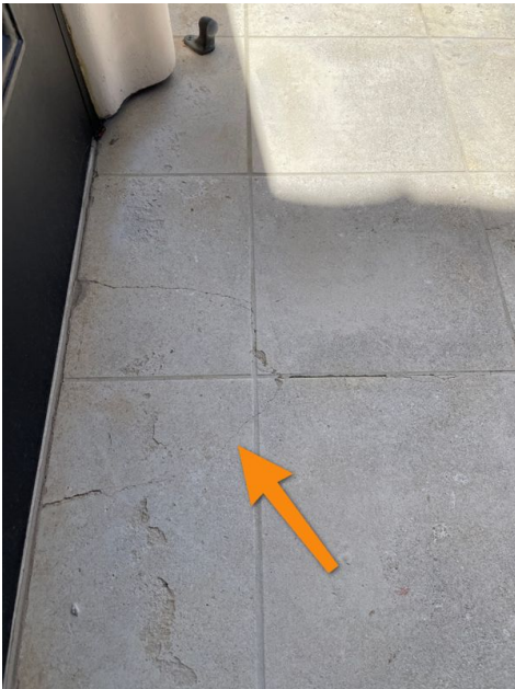
Example Noted At Balcony
