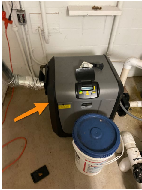
Example Noted At Pool Equipment Room
