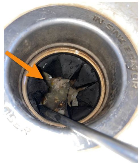
Example Noted At Pool House Kitchen
