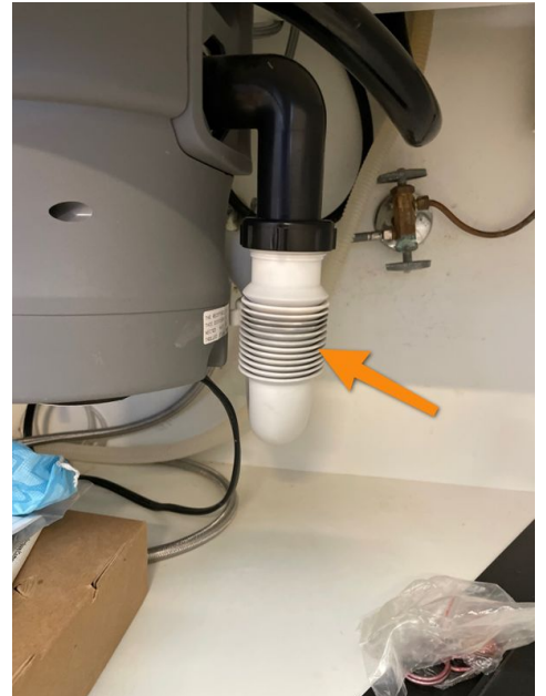
Example Noted At Kitchen Casita/Granny Flat
