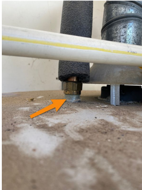
Example Noted At Pool House
