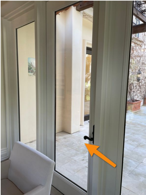
Example Noted At Kitchen Dining Room
