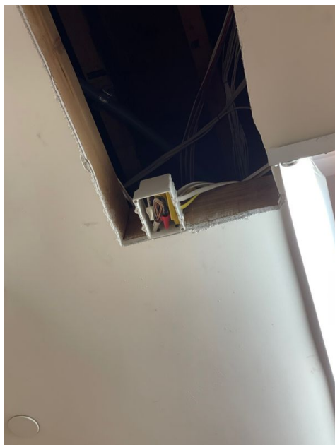
Example Noted At Basement
