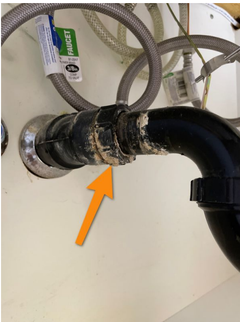
Example Noted At Master Bathroom Casita/Granny Flat
