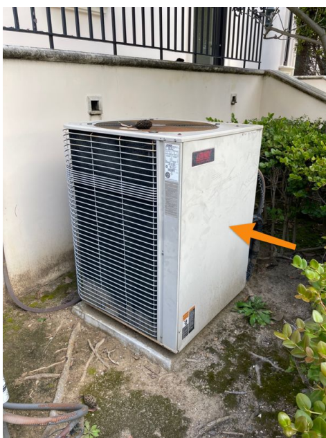
Example Noted At Right Side Of Home
