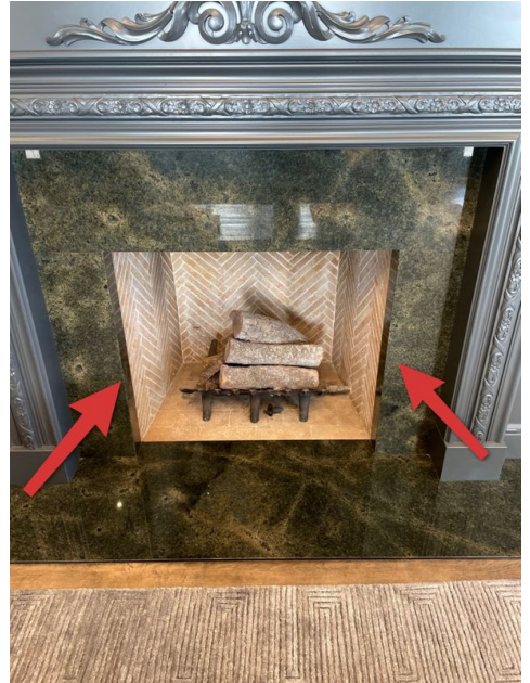
Example Noted At Office
