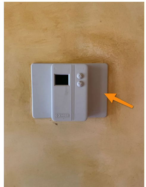
Example Noted At Wine Room
