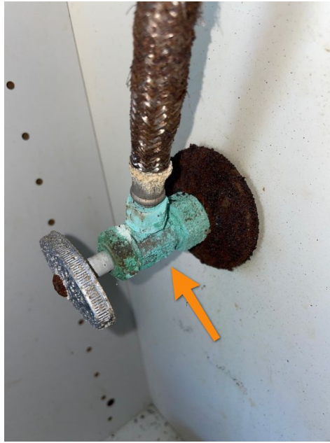
Example Noted At Garage
