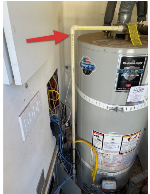
Example Noted At Pool House
