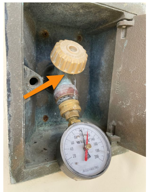
Example Noted At Balcony
