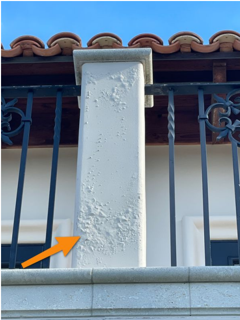
Example Noted At Rear Side Of Home
