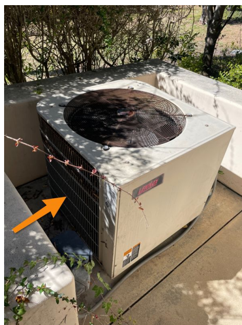
Example Noted At Pool House
