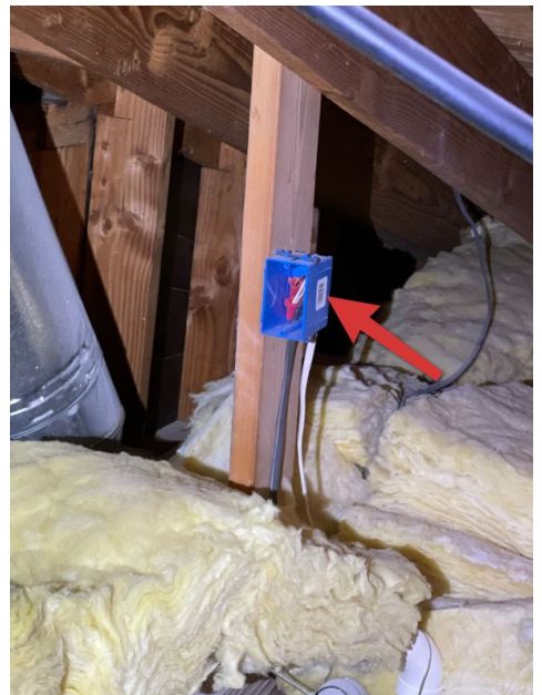
Example Noted At Attic
