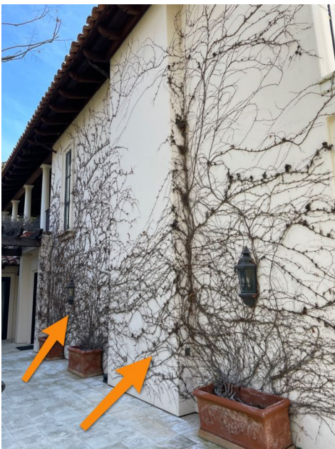
Example Noted At Left Side Of Home
