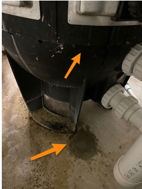
Example Noted At Pool Equipment Room
