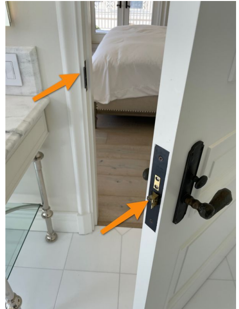
Example Noted At Bedroom 4 Bathroom
