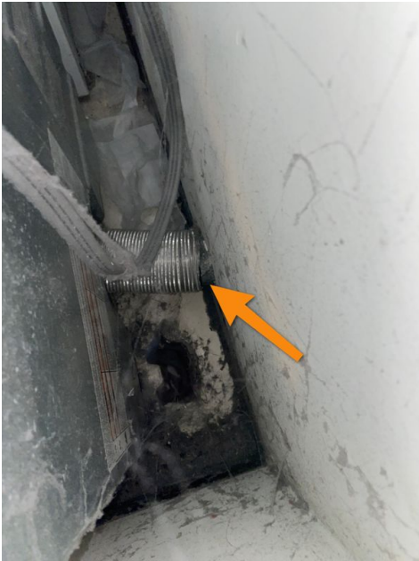
Example Noted At Garage
