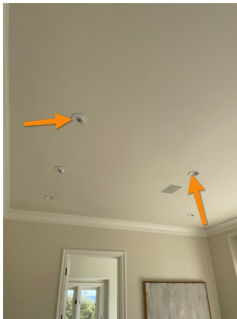
Example Noted At Bedroom 4
