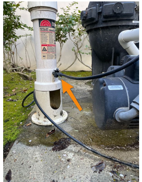
Example Noted At Pool Equipment Right Side Of Home
