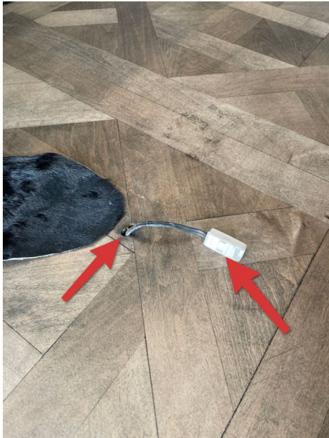
Example Noted At Office
