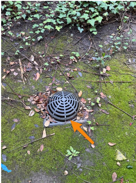
Example Noted At Left Side Of Home
