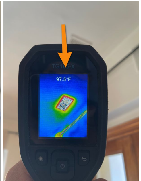
Example Noted At Pool House
