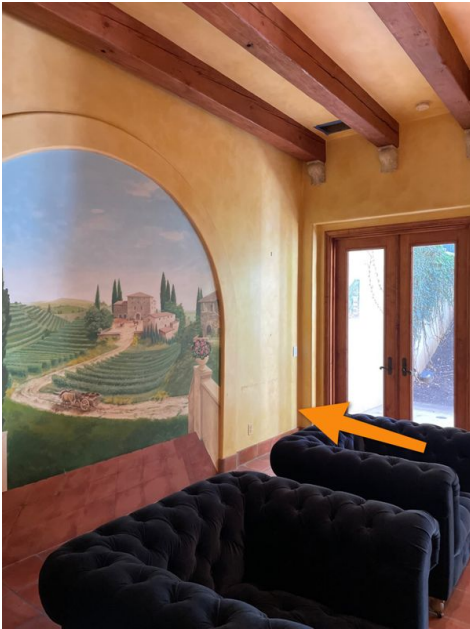
Example Noted At Wine Room
