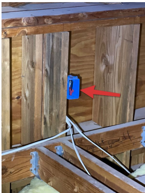
Example Noted At Attic
