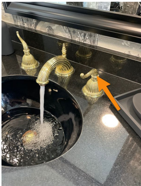
Example Noted At Guest Bathroom
