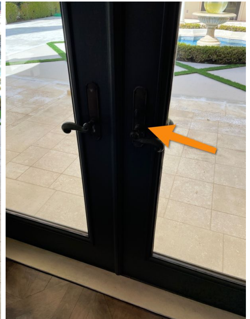
Example Noted At Office
