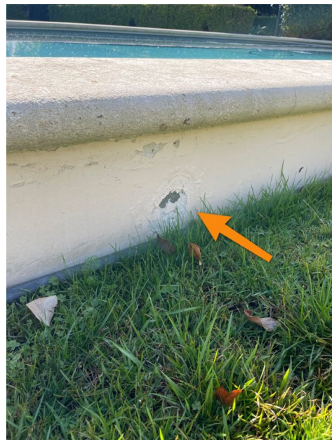
Example Noted At Pool
