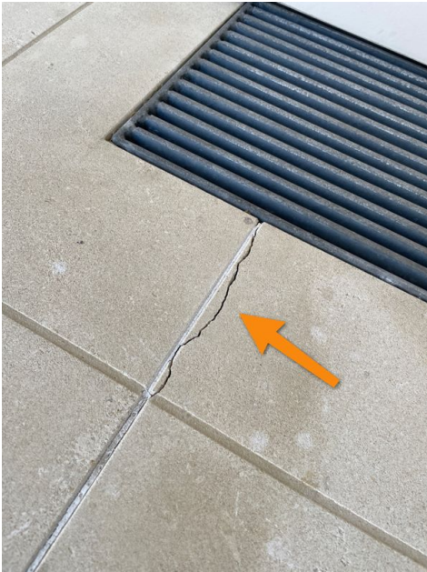
Example Noted At Rear Side Of Home
