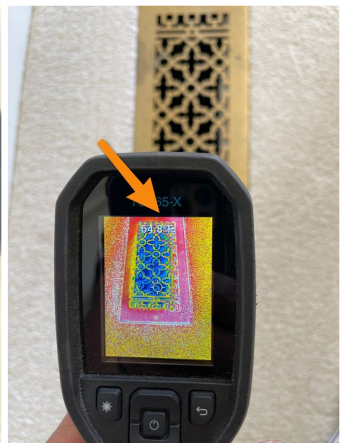
Example Noted At Bedroom 5
