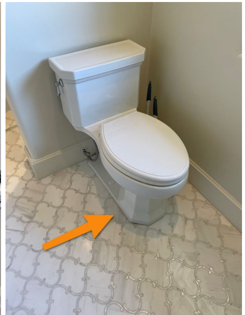
Example Noted At Master Bathroom Casita/Granny Flat
