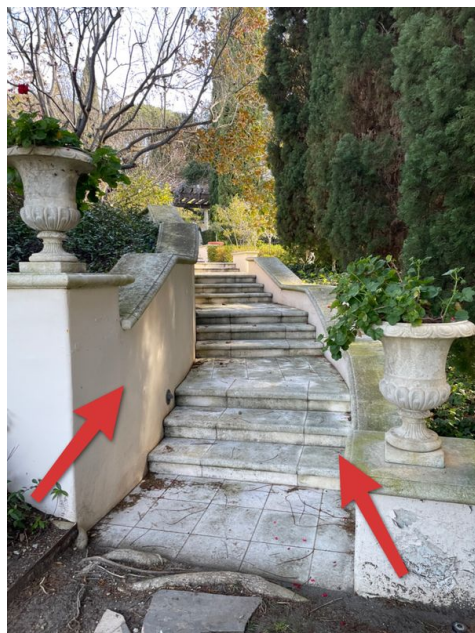
Example Noted At Right Side Of Home
