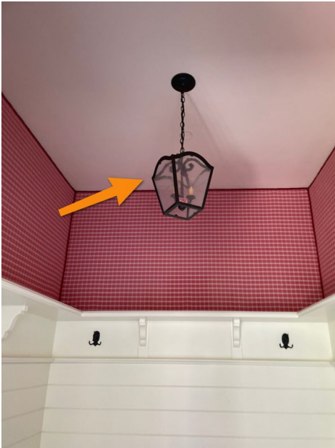
Example Noted At Second Story Exterior Closet Left Side Of Home
