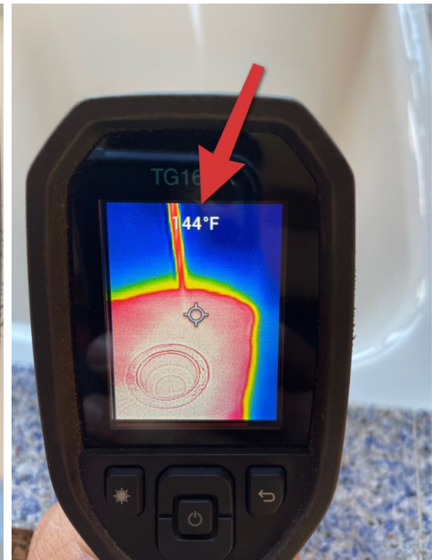
Example Noted At Pool House Kitchen
