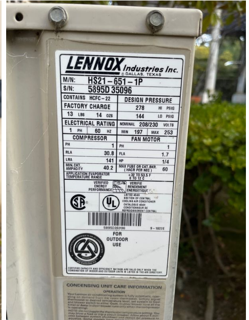
Example Noted At Right Side Of Home
