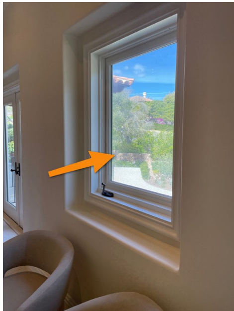
Example Noted At Bedroom 2
