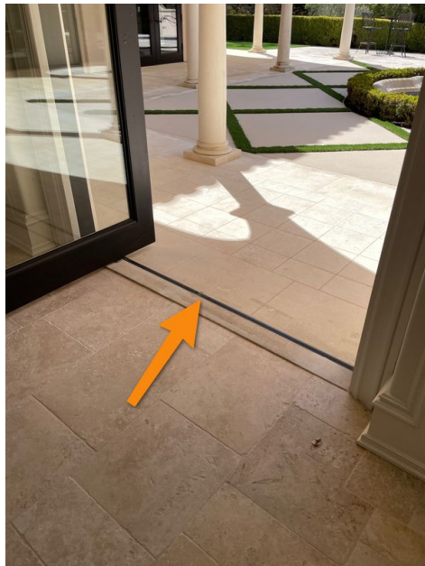
Example Noted At Rear Side Of Home
