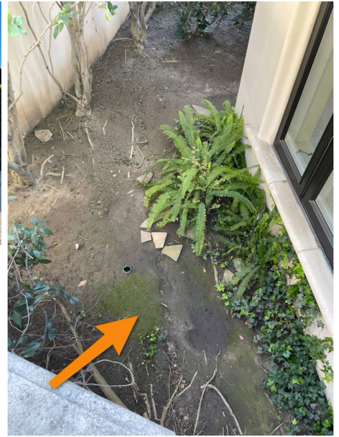
Example Noted At Left Side Of Home
