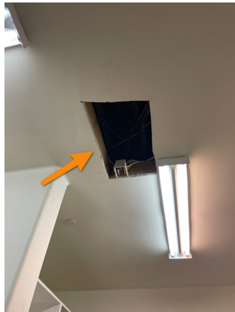
Example Noted At Basement
