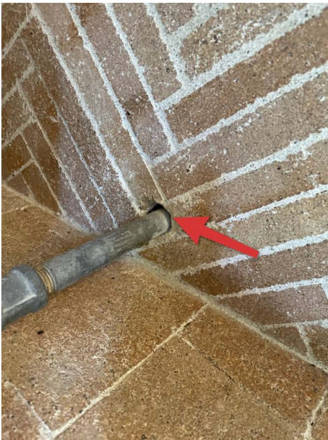
Example Noted At Living Room
