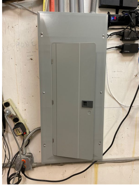
Example Noted At Basement
