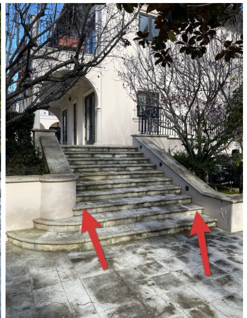
Example Noted At Right Side Of Home
