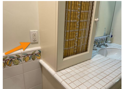
Example Noted At Pool House Bathroom
