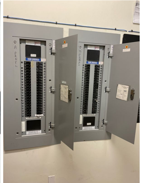
Example Noted At Basement
