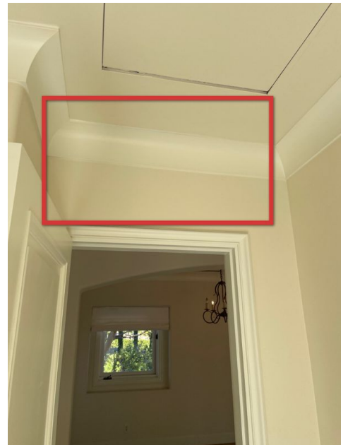
Example Noted At Bedroom 2 Casita/Granny Flat
