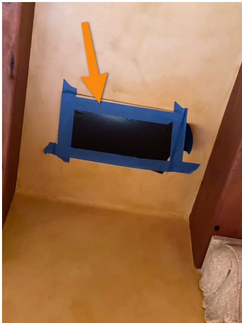
Example Noted At Wine Room
