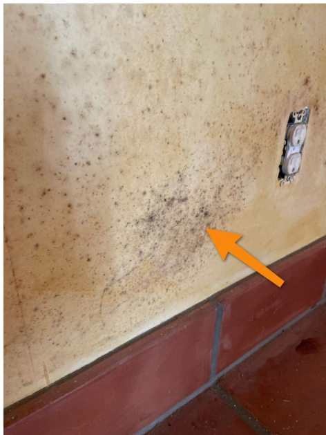
Example Noted At Wine Room
