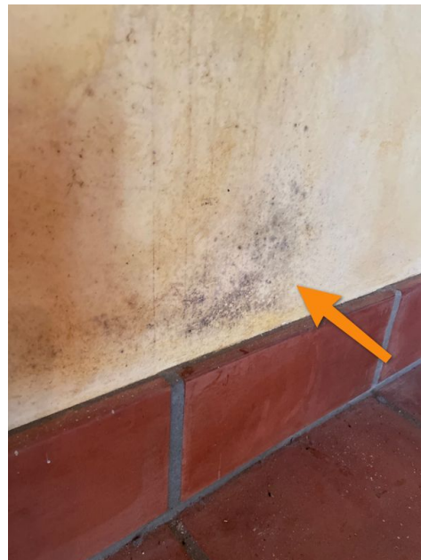
Example Noted At Wine Room
