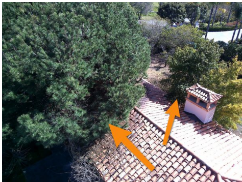
Example Noted At Pool House
