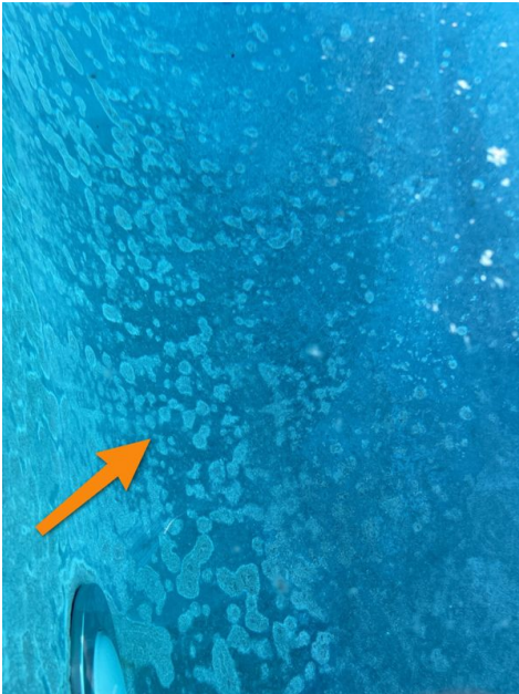
Example Noted At Pool
