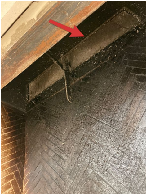
Example Noted At Dining Room
