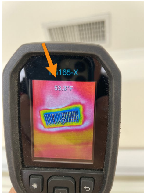
Example Noted At Bedroom 2 Casita/Granny Flat
