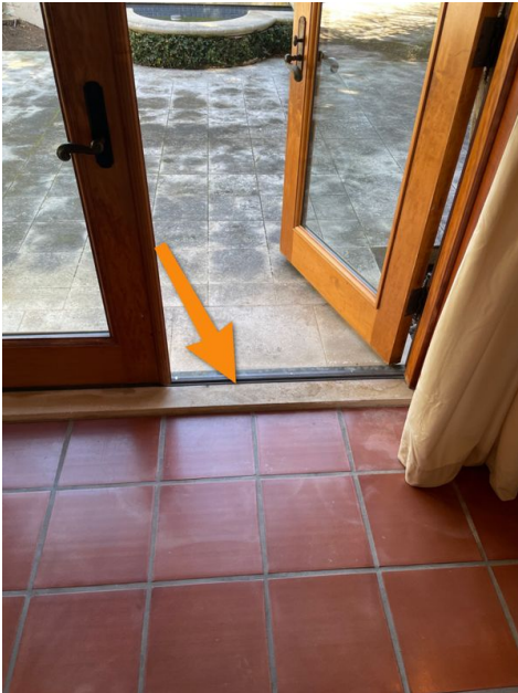
Example Noted At Pool house
