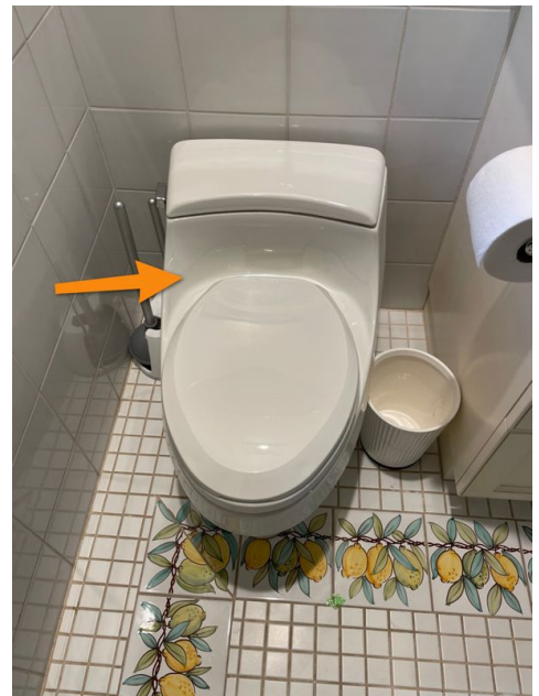
Example Noted At Pool House Bathroom
