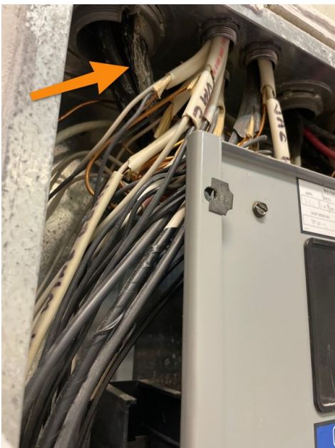
Example Noted At B Sub Panel
