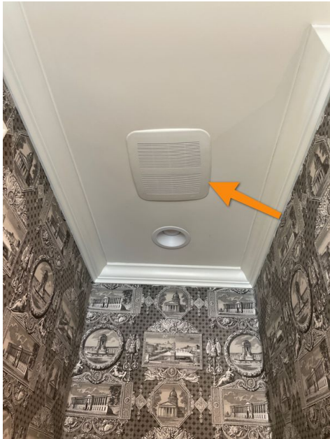
Example Noted At Guest Bathroom
