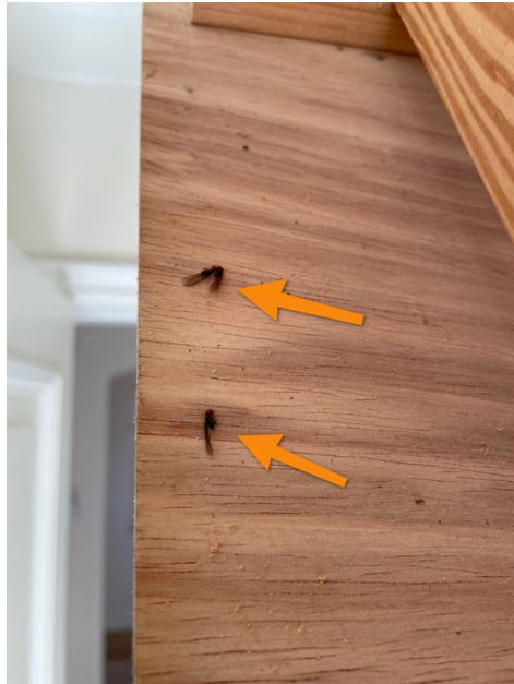
Example Noted At Casita/Granny Flat Attic
