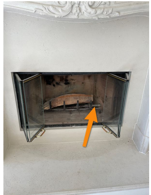
Example Noted At Casita/Granny Flat
