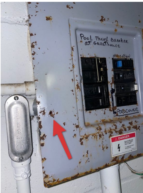
Example Noted At Pool Equipment Room
