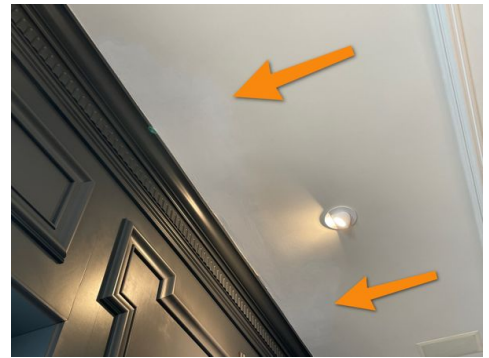
Example Noted At Office
