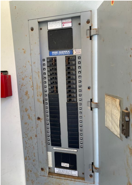
Example Noted At Pool House
