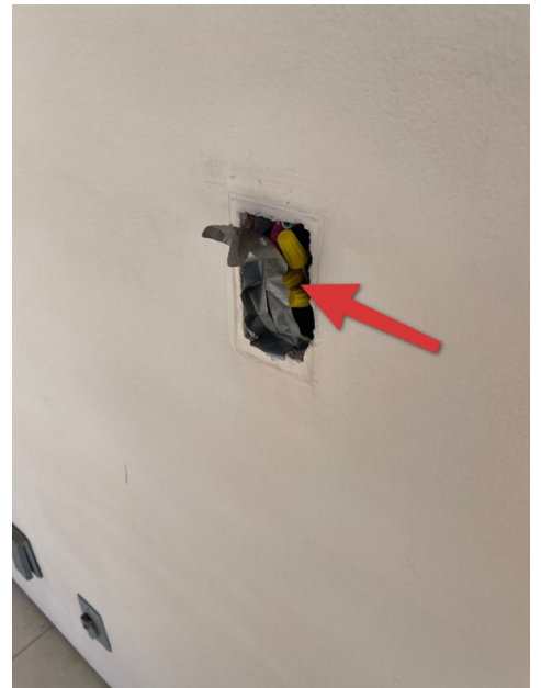
Example Noted At Rear Side Of Home Balcony
