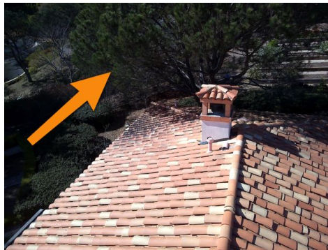
Example Noted At Garage
