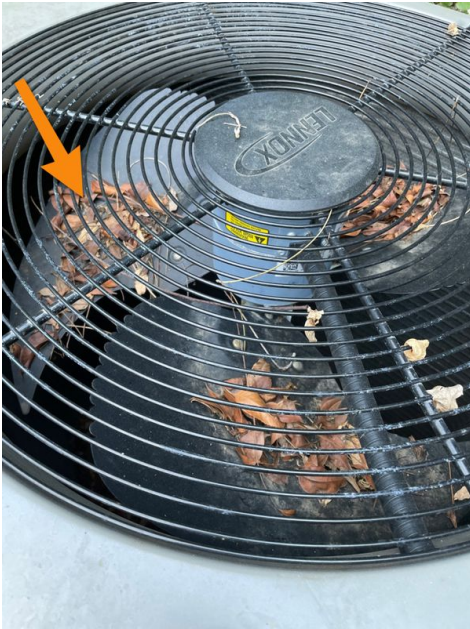
Example Noted At Left Side Of Home
