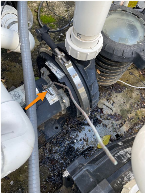
Example Noted At Pool Equipment Right Side Of Home
