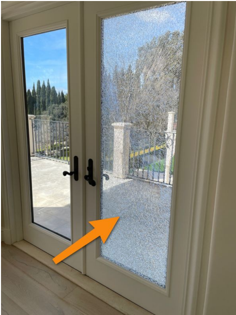
Example Noted At Bedroom 4
