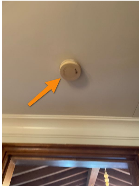
Example Noted At Pool House Bedroom
