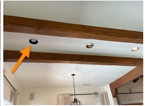
Example Noted At Pool House Kitchen
