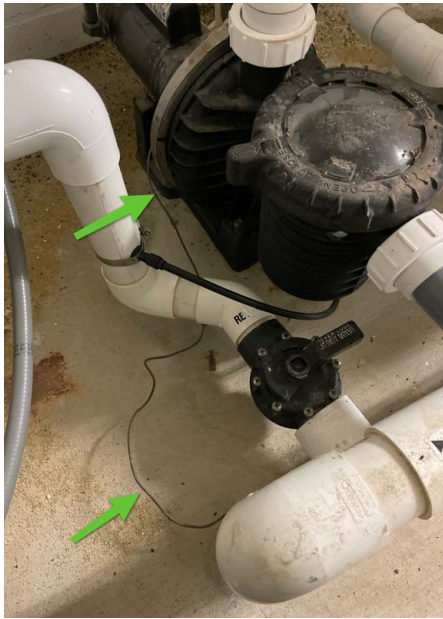
Example Noted At Pool Equipment Room
