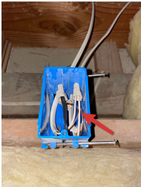
Example Noted At Attic
