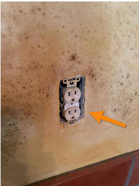
Example Noted At wine Room
