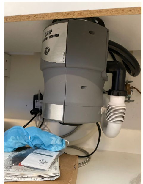
Example Noted At Casita/Granny Flat
