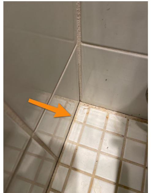
Example Noted At Pool House Bathroom
