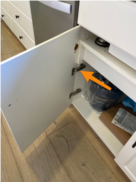
Example Noted At Kitchen Casita/Granny Flat
