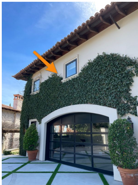
Example Noted At Garage
