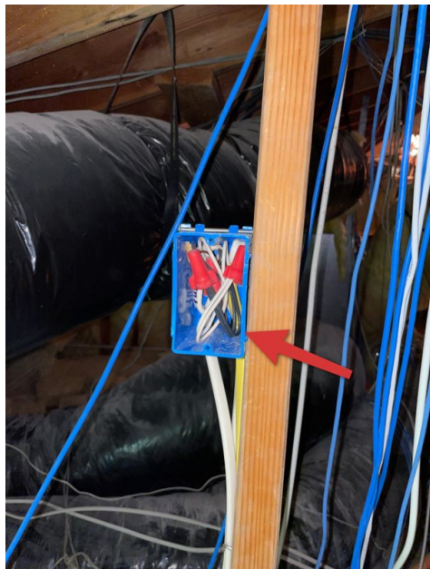
Example Noted At Attic
