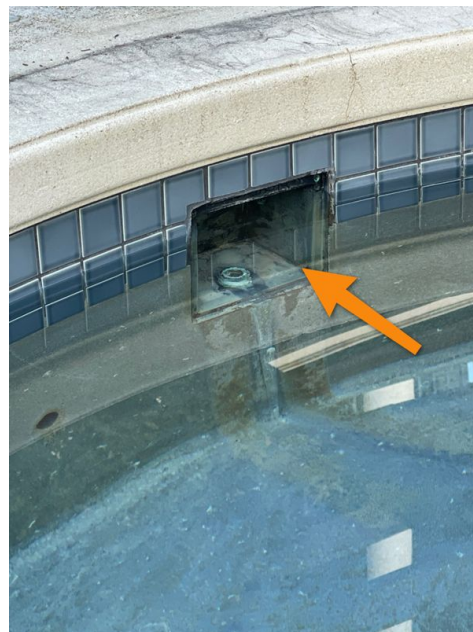
Example Noted At Spa Right Side Of Home
