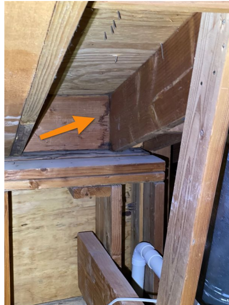
Example Noted At Attic
