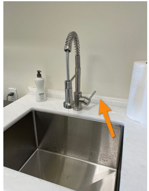
Example Noted At Laundry Room
