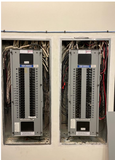
Example Noted At Basement
