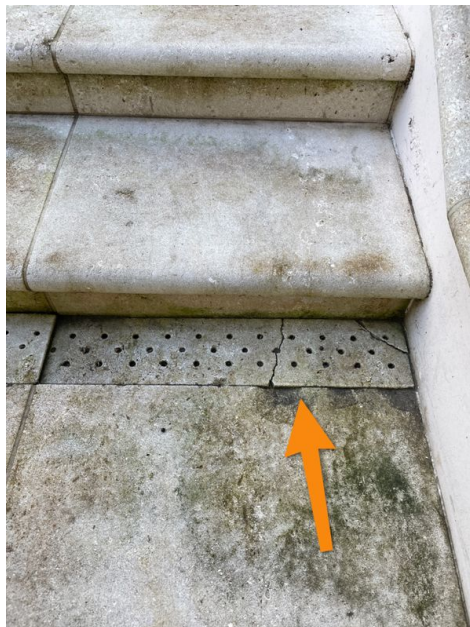
Example Noted At Left Side Of Home
