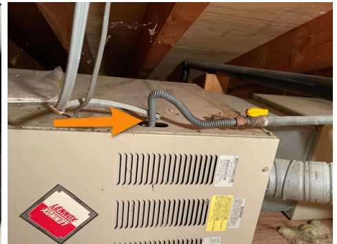
Example Noted At Pool House
