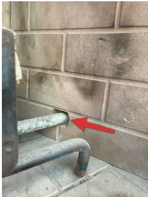
Example Noted At Casita/Granny Flat
