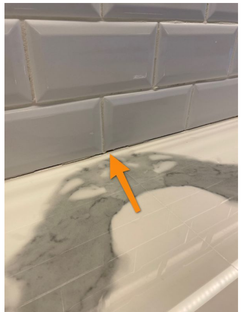
Example Noted At Kitchen Casita/Granny Flat
