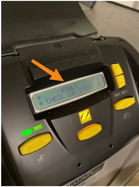
Example Noted At Pool Equipment Room
