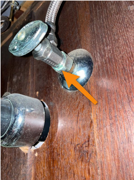
Example Noted At Guest Bathroom
