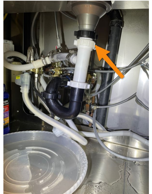
Example Noted At Kitchen
