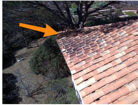
Example Noted At Garage
