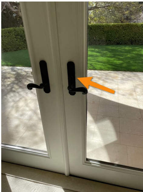
Example Noted At Bedroom 5
