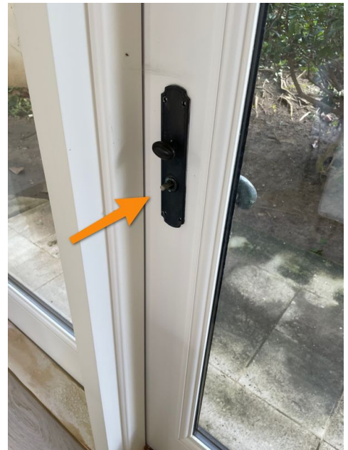
Example Noted At Dining Room
