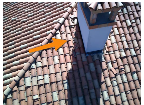
Example Noted At Roof
