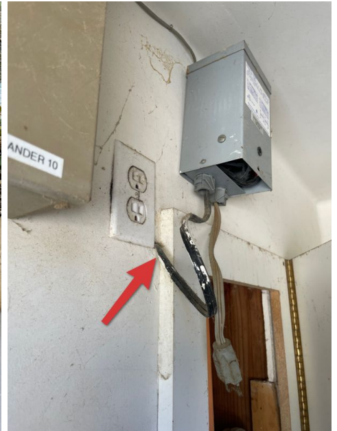
Example Noted At Pool House Water Heater Closet
