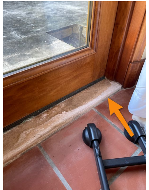
Example Noted At Pool House Living Room
