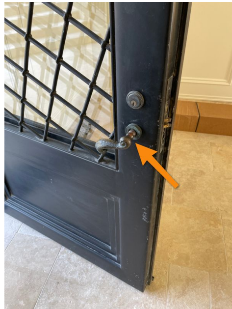
Example Noted At Front Entrance
