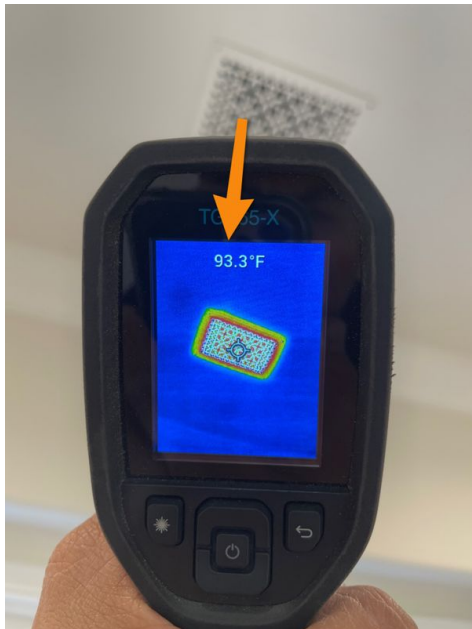
Example Noted At Bedroom 3
