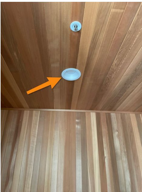
Example Noted At Gym Sauna
