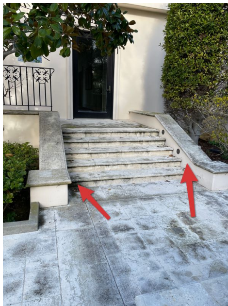
Example Noted At Right Side Of Home
