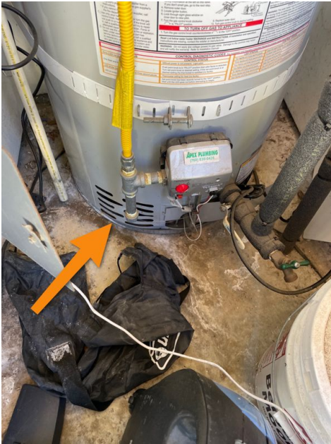
Example Noted At Pool House
