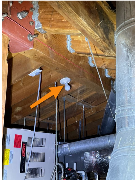
Example Noted At Casita/Granny Flat Attic
