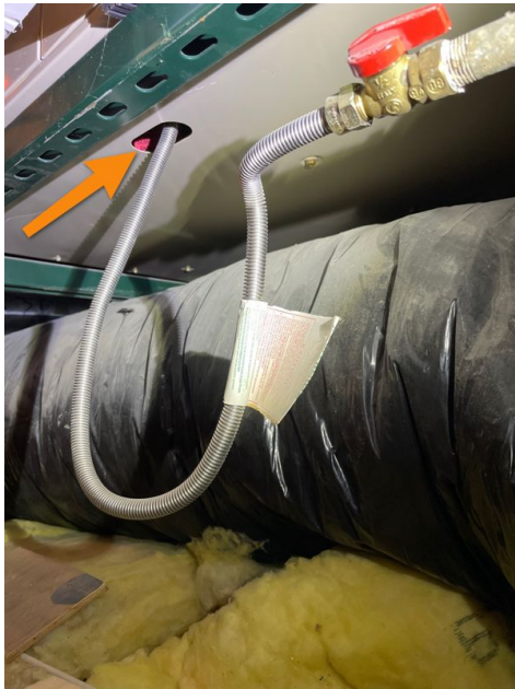
Example Noted At Furnace
