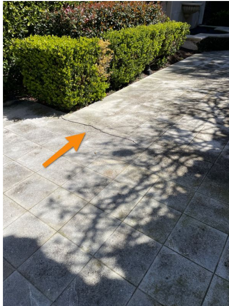
Example Noted At Pool House
