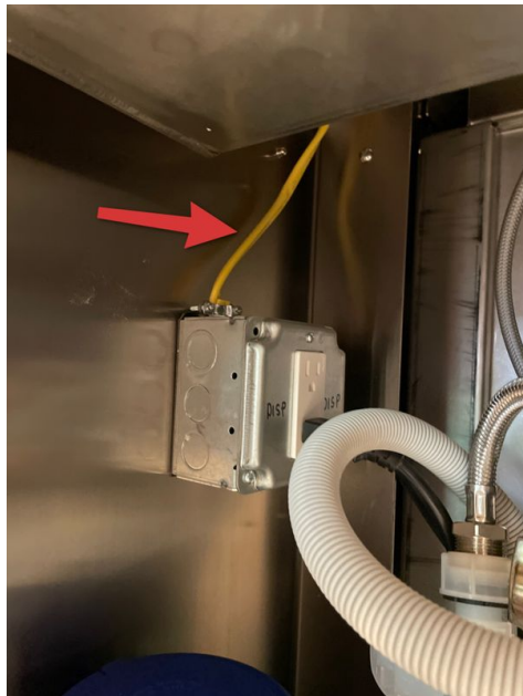
Example Noted At Kitchen
