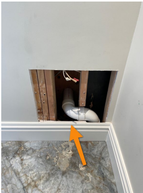
Example Noted At Kitchen Closet
