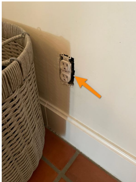
Example Noted At Pool House Bedroom
