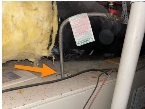
Example Noted At Crawlspace
