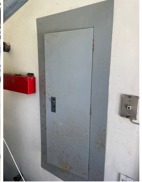
Example Noted At Pool House
