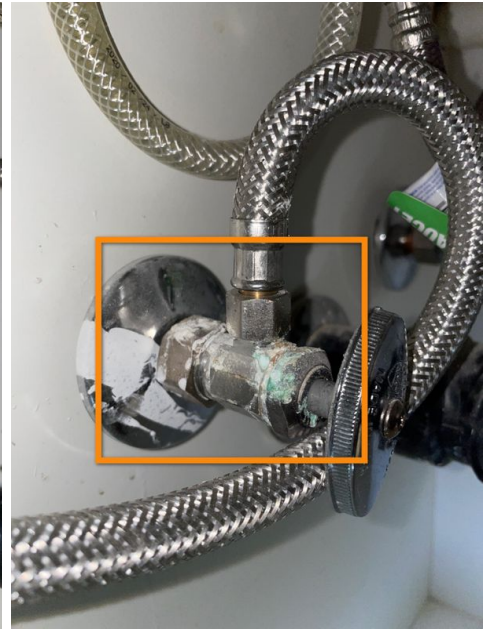
Example Noted At Hallway Bathroom Casita/Granny Flat
