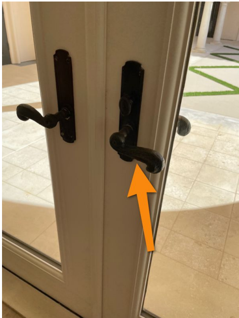
Example Noted At Dining Room
