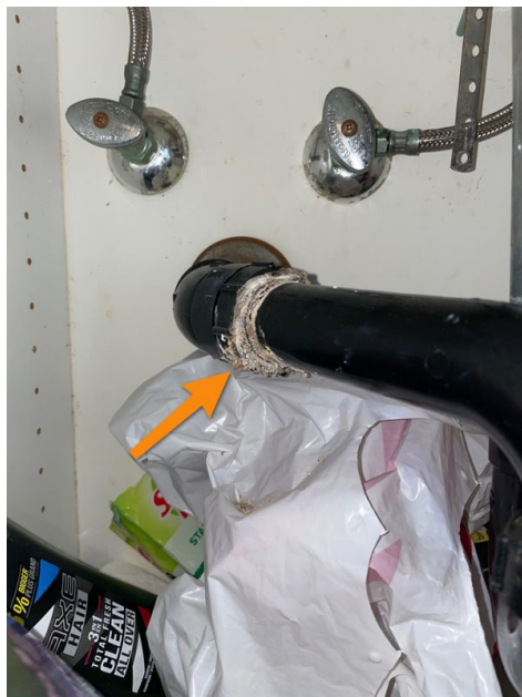
Example Noted At Pool House Bathroom
