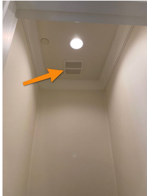
Example Noted At Master Bathroom
