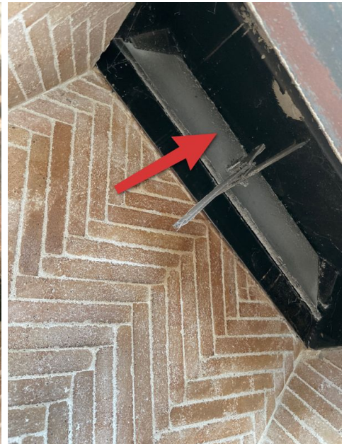
Example Noted At Master Bedroom
