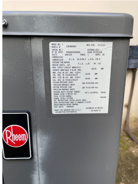
Example Noted At Right Side Of Home
