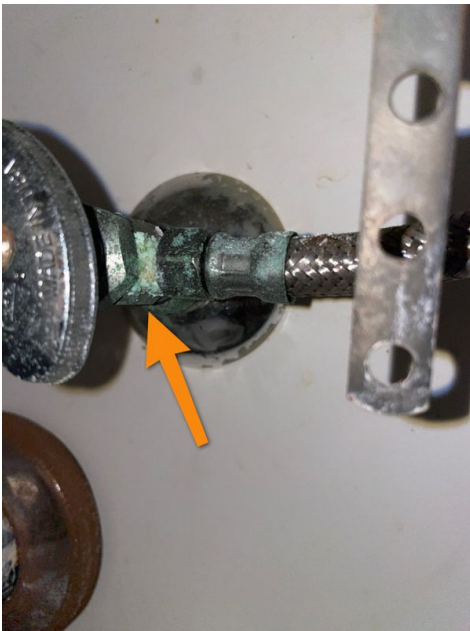
Example Noted At Pool House Bathroom
