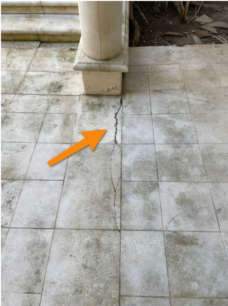
Example Noted At Left Side Of Home
