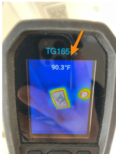
Example Noted At Master Bedroom
