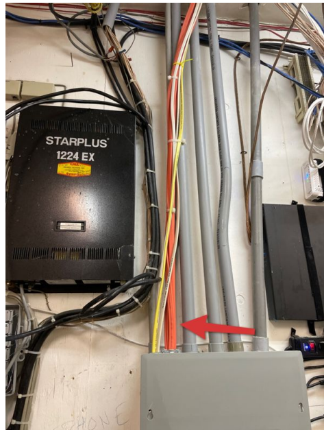
Example Noted At Basement
