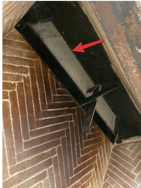
Example Noted At Living Room
