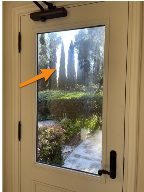
Example Noted At Casita/Granny Flat
