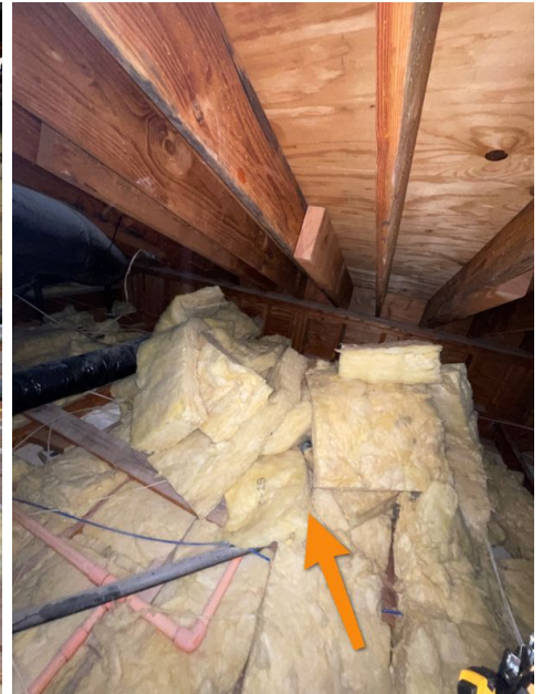
Example Noted At Attic
