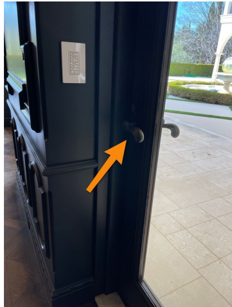
Example Noted At Office
