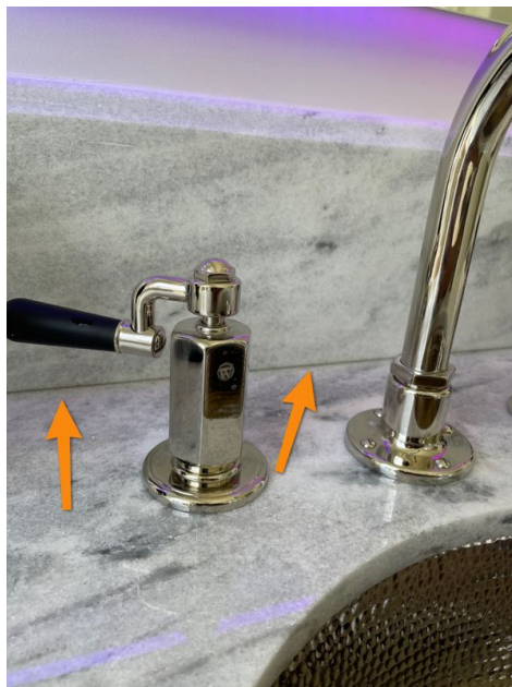
Example Noted At Bedroom 4 Bathroom
