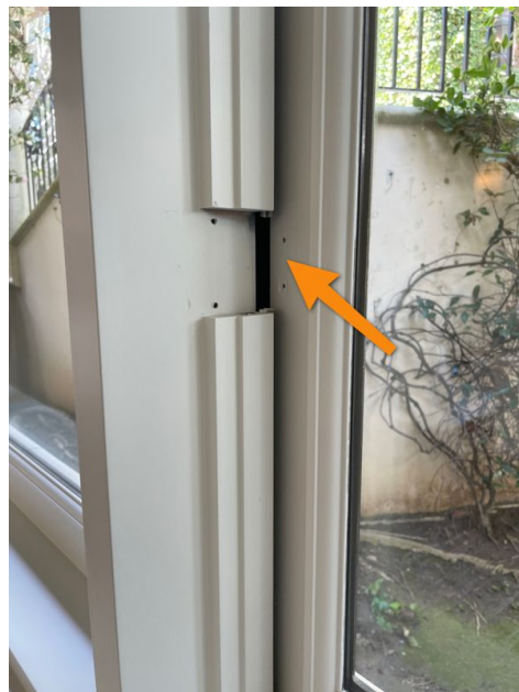
Example Noted At Dining Room
