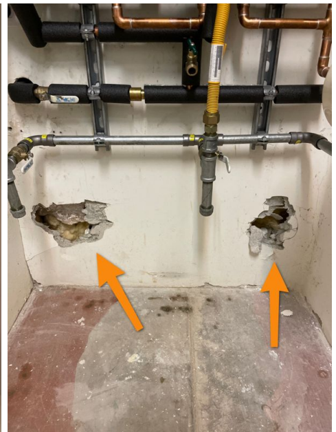
Example Noted At Basement
