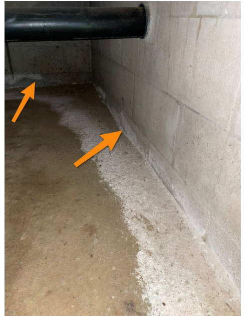
Example Noted At Crawlspace
