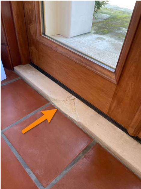
Example Noted At Pool House Dining Room
