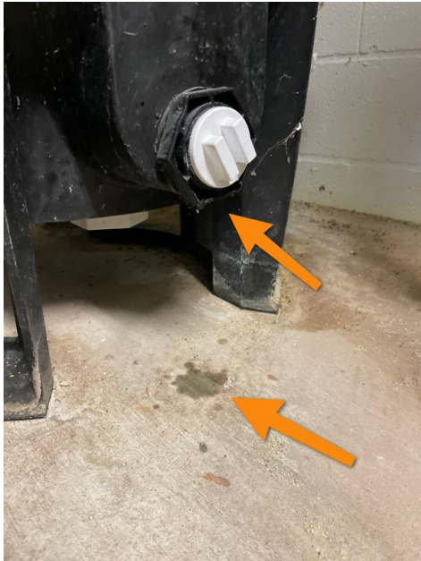
Example Noted At Pool Equipment Room
