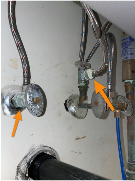
Example Noted At Laundry Room
