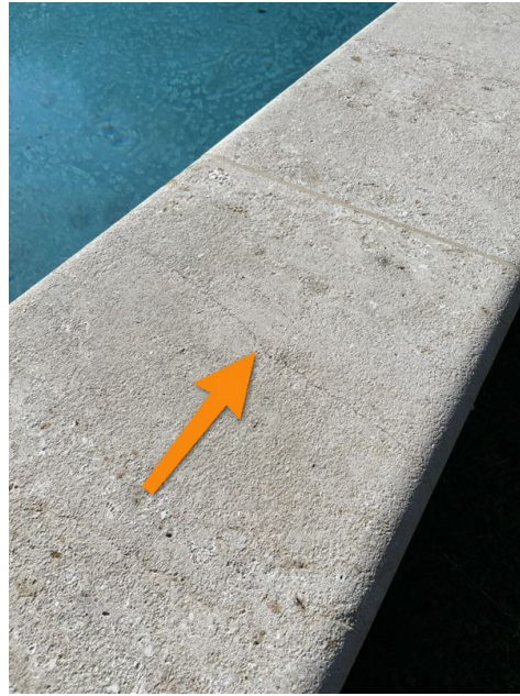
Example Noted At Pool
