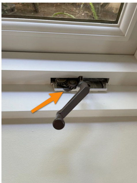
Example Noted At Dining Room
