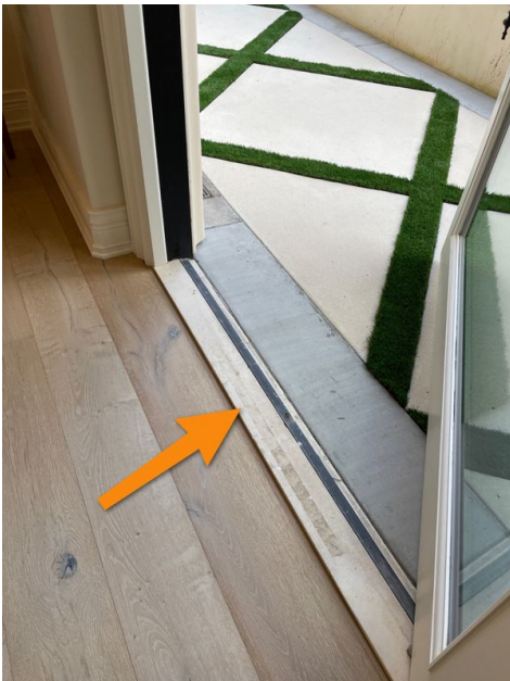
Example Noted At Living Room
