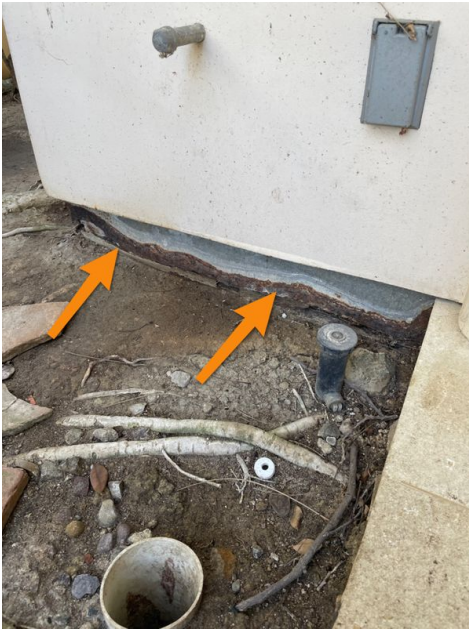
Example Noted At Left Side Of Home
