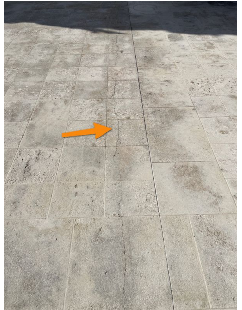
Example Noted At Rear Side Of Home
