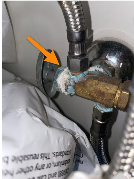
Example Noted At Pool House Kitchen
