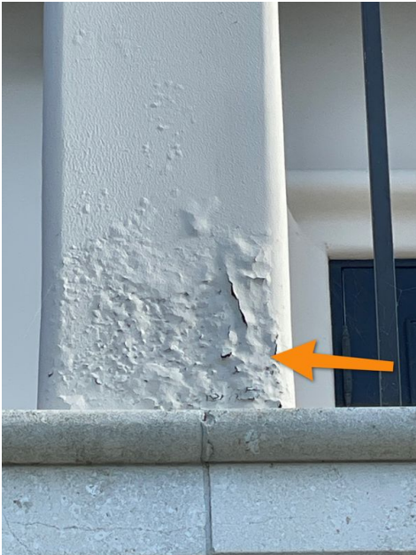
Example Noted At Balcony Rear Side Of Home
