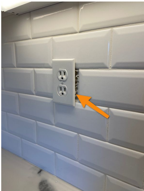
Example Noted At Kitchen Casita/Granny Flat
