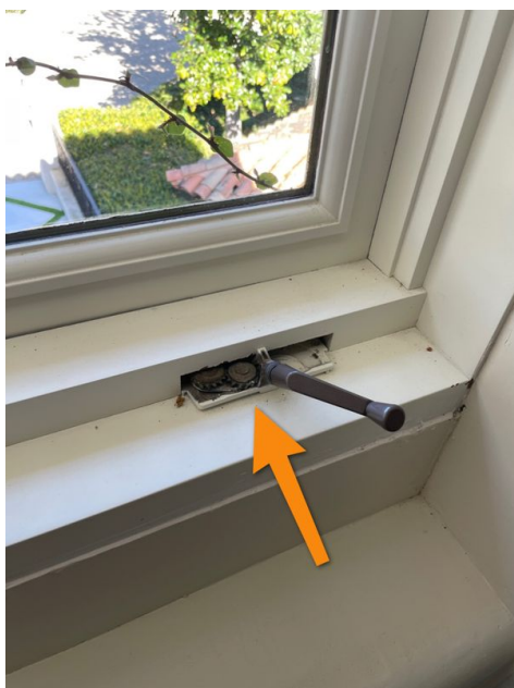
Example Noted At Master Bathroom Casita/Granny Flat
