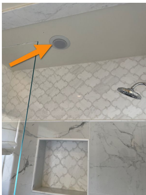
Example Noted At Master Bathroom Casita/Granny Flat
