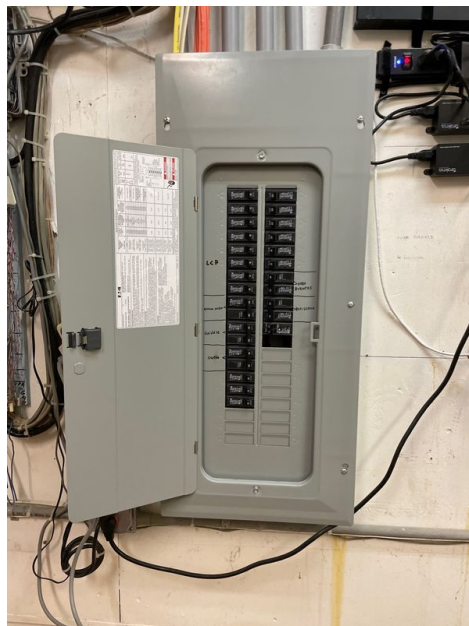
Example Noted At Basement
