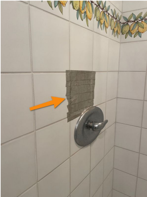
Example Noted At Pool House Bathroom
