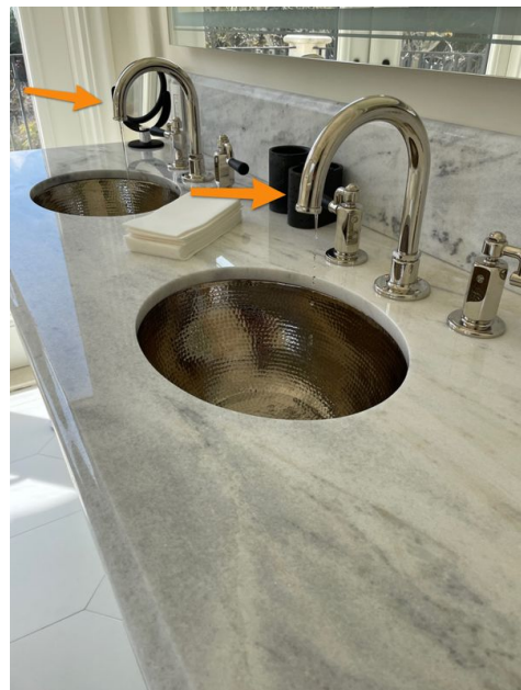
Example Noted At Bedroom 4 Bathroom
