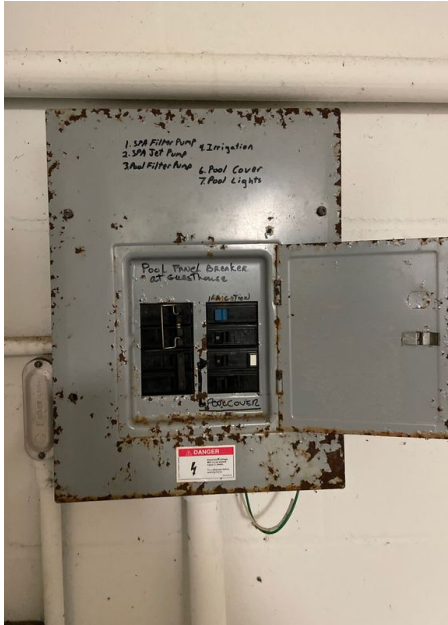
Example Noted At Pool Equipment Room
