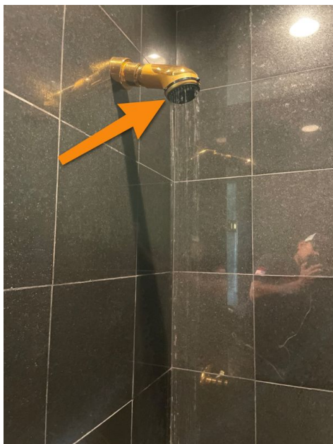
Example Noted At Guest Bathroom
