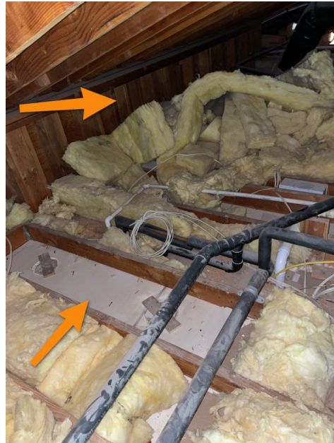
Example Noted At Attic
