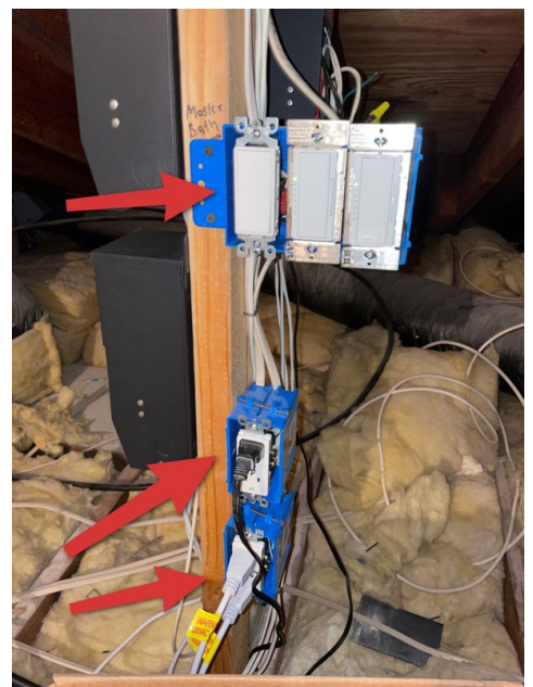
Example Noted At Attic
