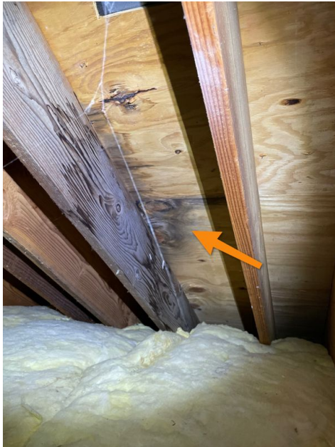
Example Noted At Attic
