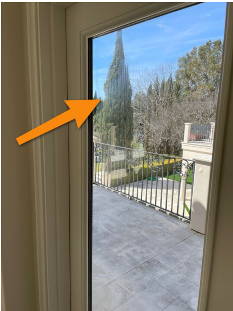
Example Noted At Bedroom 4
