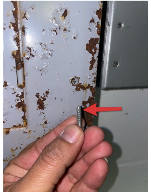
Example Noted At Pool Equipment Room
