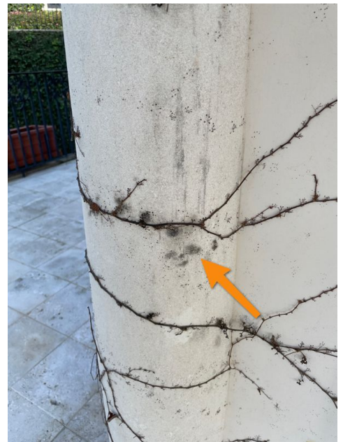
Example Noted At Rear Side Of Home
