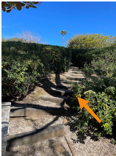
Example Noted At Left Side Of Home
