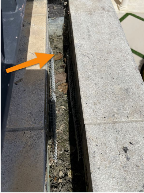
Example Noted At Balcony
