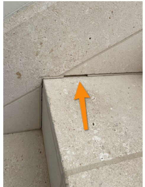
Example Noted At Casita/Granny Flat Stairs
