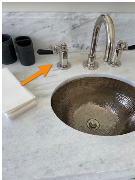
Example Noted At Bedroom 4 Bathroom
