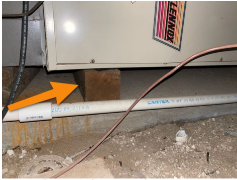
Example Noted At Crawlspace
