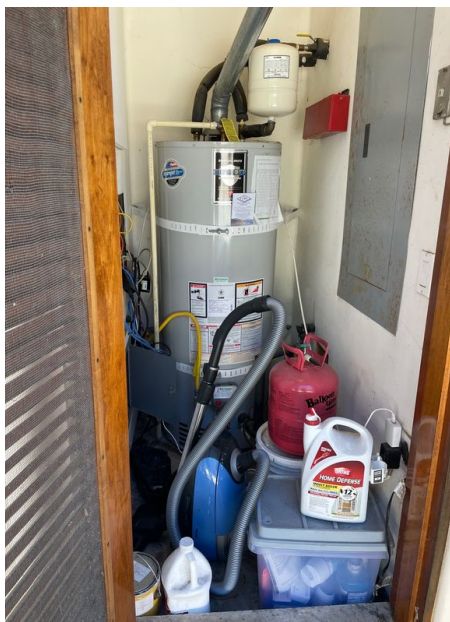
Example Noted At Pool House
