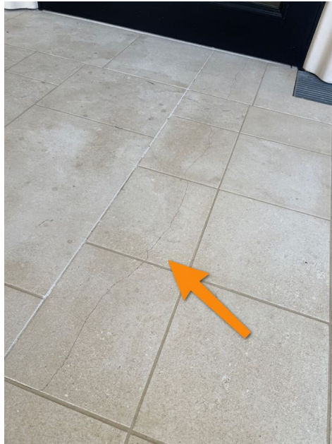
Example Noted At Rear Side Of Home
