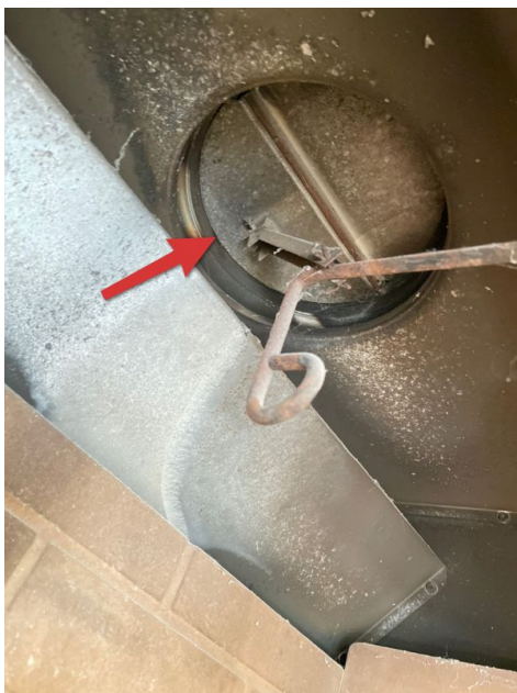
Example Noted At Casita/Granny Flat
