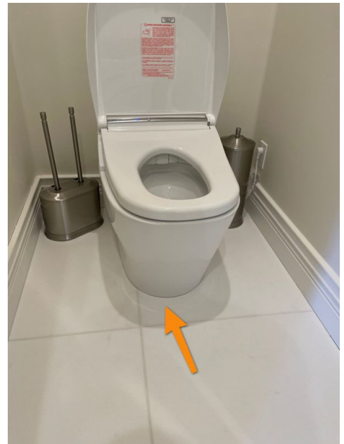
Example Noted At Master Bathroom
