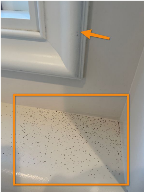
Example Noted At Hallway Bathroom Casita/Granny Flat
