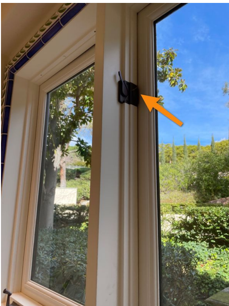
Example Noted At Kitchen Closet
