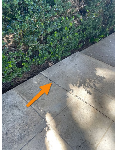
Example Noted At Pool House
