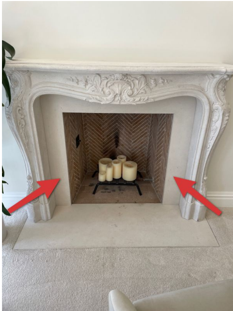
Example Noted At Master Bedroom
