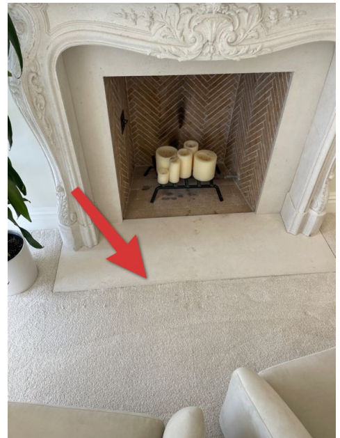
Example Noted At Master Bedroom
