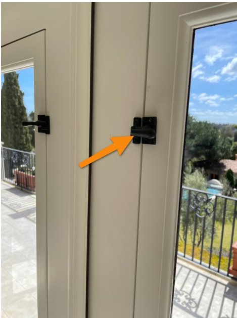
Example Noted At Master Bedroom
