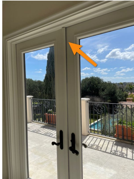
Example Noted At Master Bedroom
