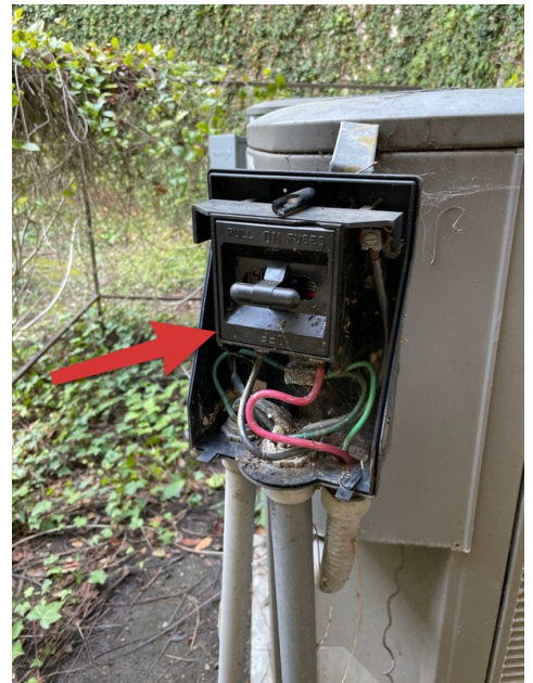
Example Noted At Left Side Of Home
