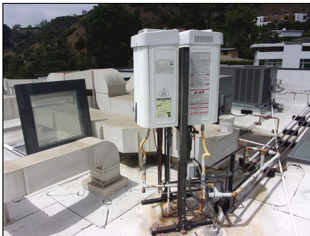
View Of Tankless Water Heaters
