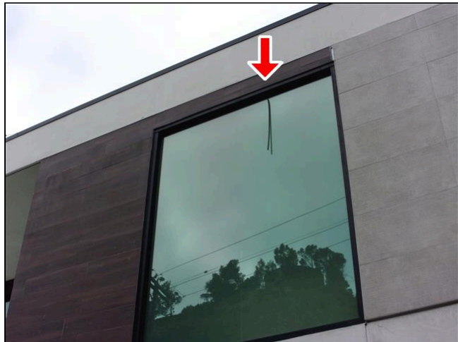
Loose Weather Stripping
