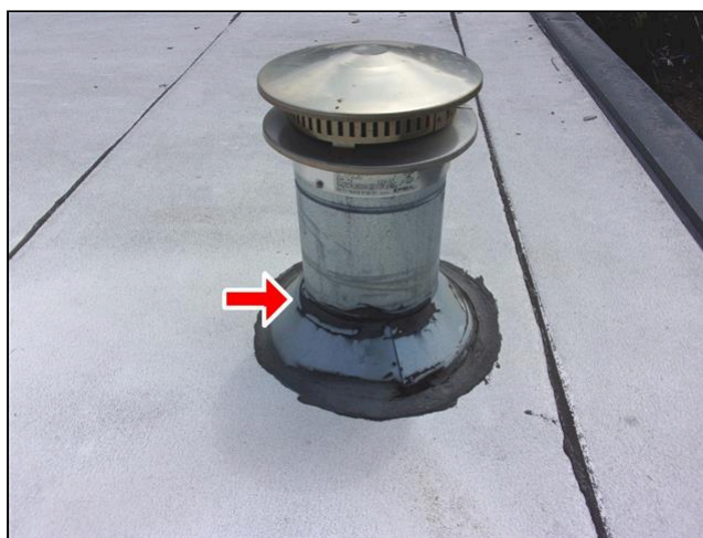
Gaps In Flashing
