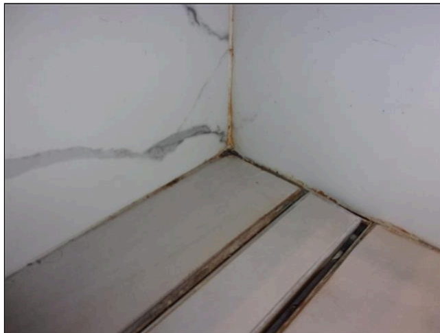
Suspected Mold/Fungus/Mildew, Front Right Bath
