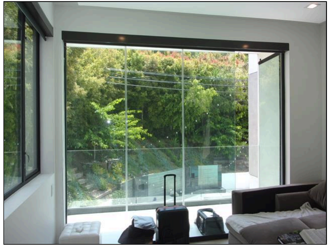
Doors Difficult To Slide
