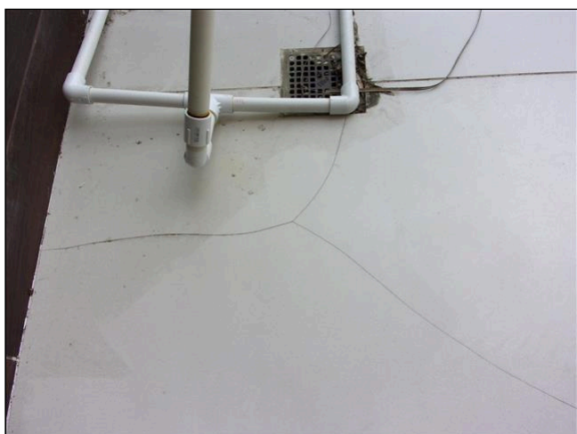
Cracked Tile Surface
