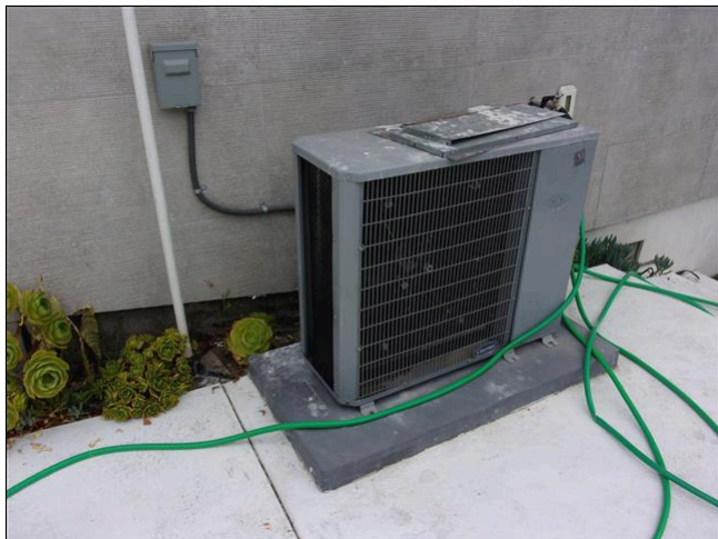
A/C Condenser View, 1st Level, Right Side
