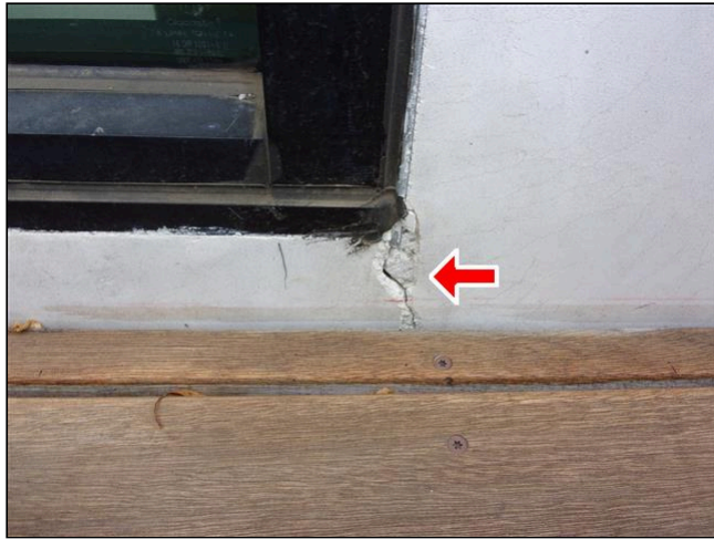
Cracked Siding, Rear Living Room Wall
