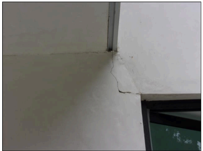
Cracked Siding, Left Side
