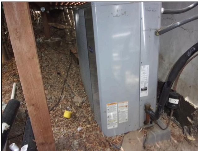
A/C Condenser View, 1st Level, Left Side
