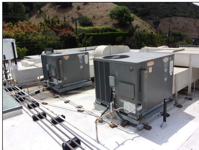
HVAC Systems Not Tested
