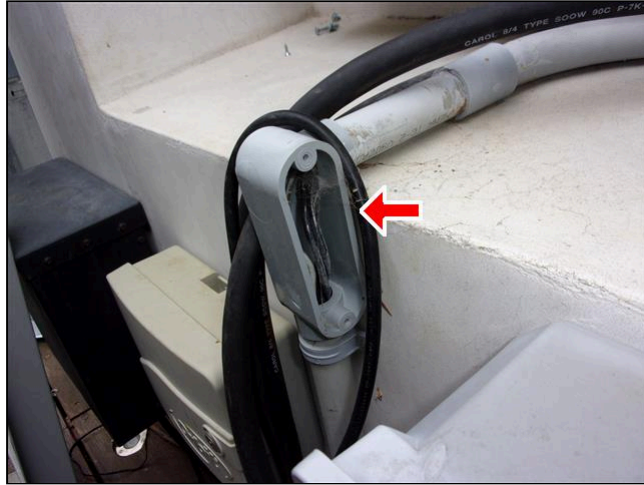
Cover Plate Missing
