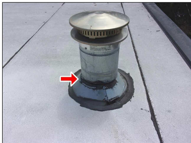
Gaps In Flashing
