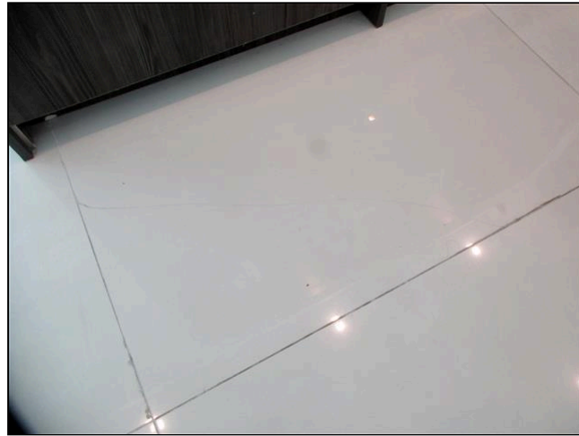
Cracked, Loose Tiles, Kitchen
