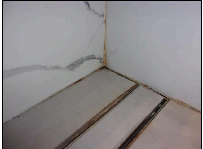
Suspected Mold/Fungus/Mildew, Front Right Bath
