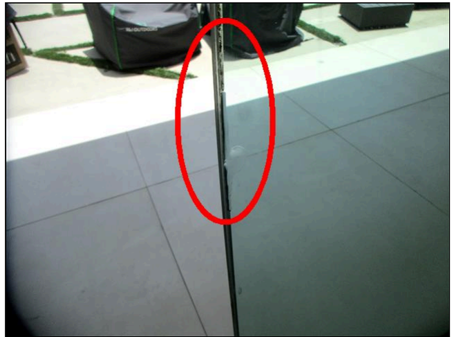
Chipped, Damaged Glass
