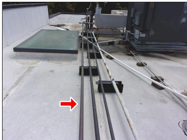
Piping Not Insulated
