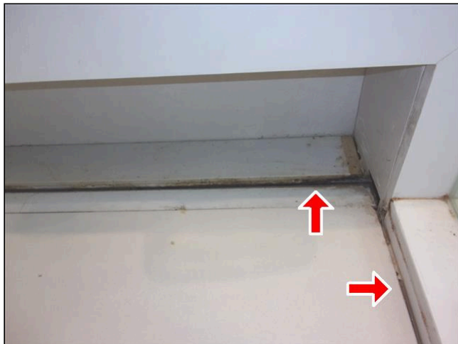
Suspected Mold/Fungus/Mildew, Front Left Guest Bath
