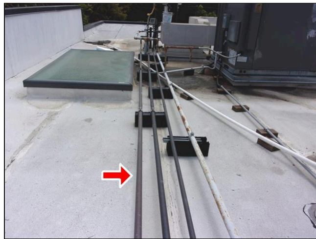
Piping Not Insulated
