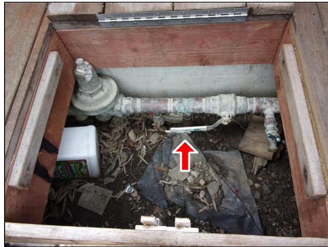
Water Shut Off Valve
