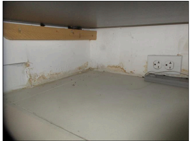
Signs Of Water Intrusion
