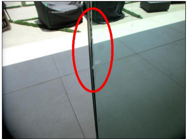
Chipped, Damaged Glass
