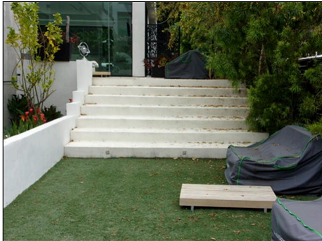
Railing Missing, Rear Steps
