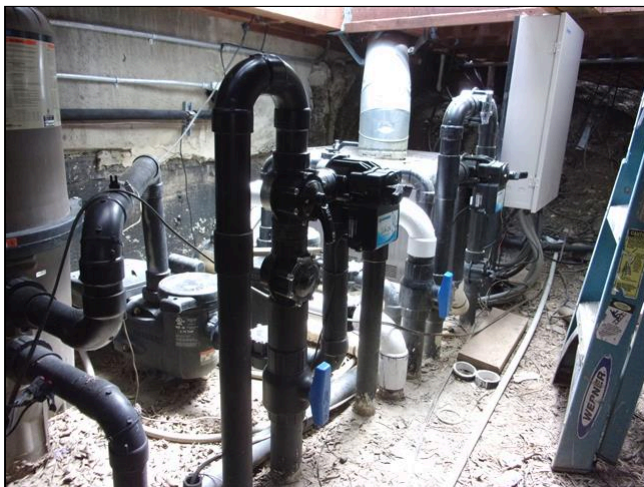
Pool/Spa Equipment View
