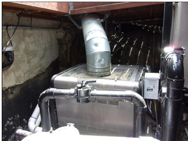
Heater Not Operational
