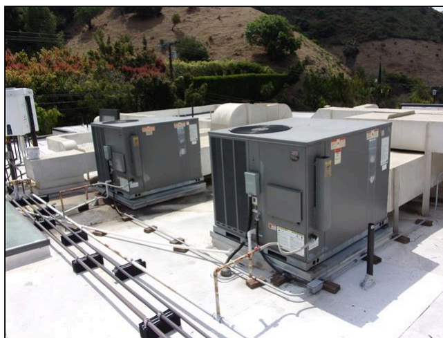
HVAC Systems Not Tested
