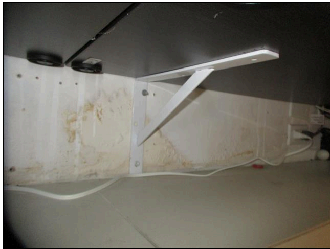
Signs Of Water Intrusion
