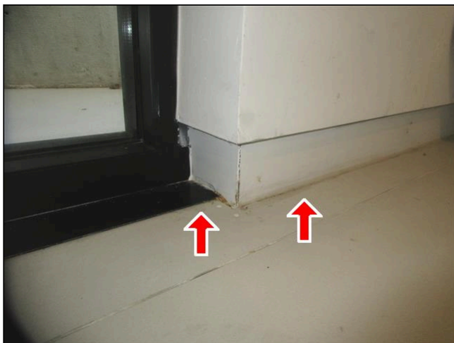
Signs Of Water Intrusion
