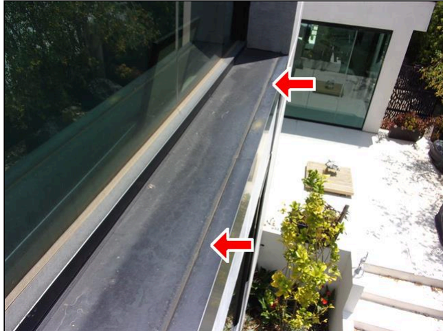
Flashing Incorrectly Sloped
