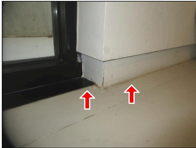
Signs Of Water Intrusion
