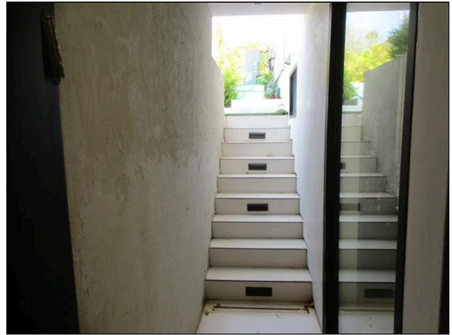
Railing Missing, Right Side Steps
