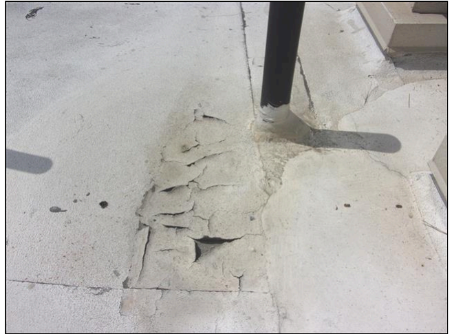
Cracked Roof Covering
