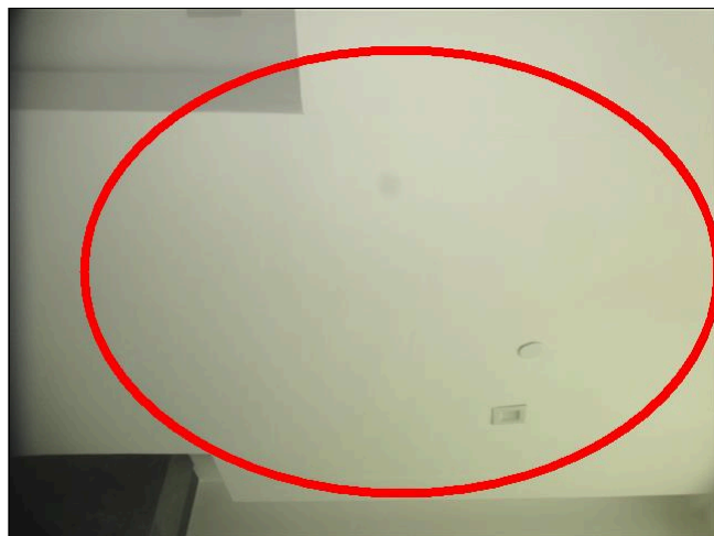
Stained, Damaged Ceiling, Living Room
