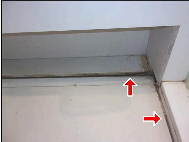
Suspected Mold/Fungus/Mildew, Front Left Guest Bath
