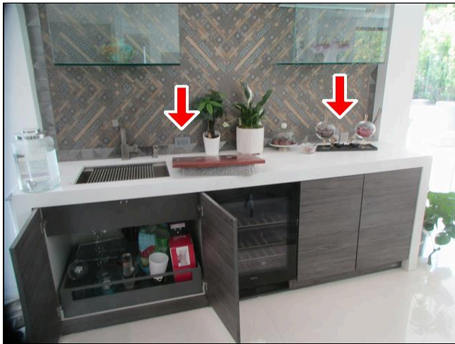
Outlets Not Operational, Kitchen
