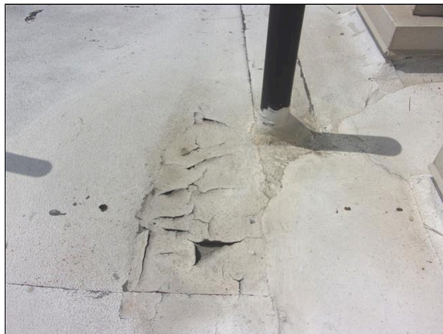
Cracked Roof Covering
