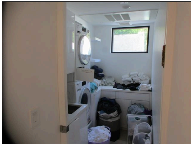
Air Handler Not Accessible
