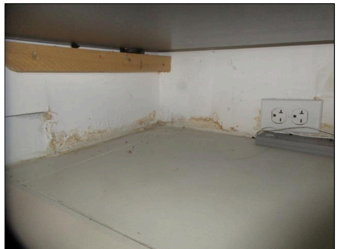
Signs Of Water Intrusion
