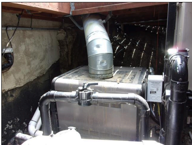
Heater Not Operational
