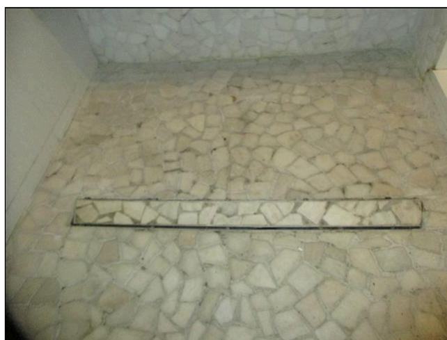
Loose Drain Cover
