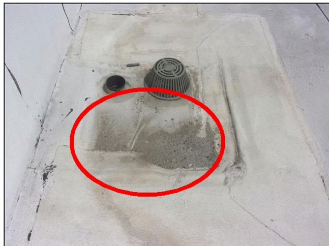
Weak Spot, Right Side Scupper
