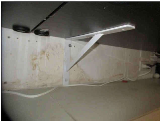
Signs Of Water Intrusion
