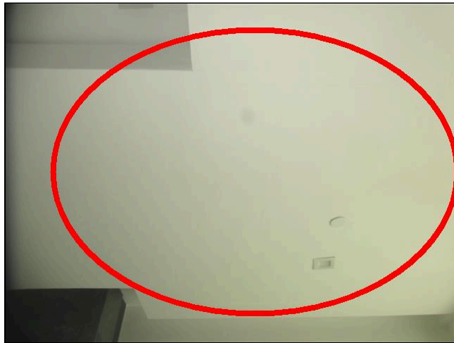
Stained, Damaged Ceiling, Living Room
