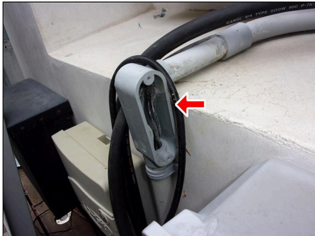
Cover Plate Missing
