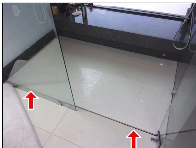
Loose Shower Pan
