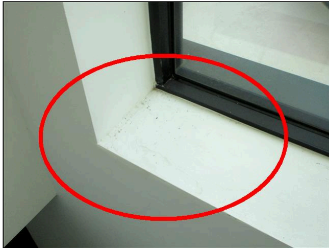
Signs Of Water Intrusion
