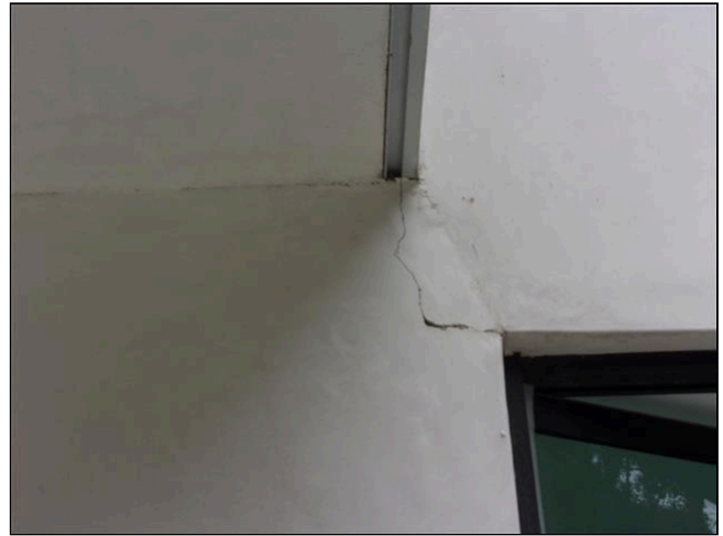
Cracked Siding, Left Side
