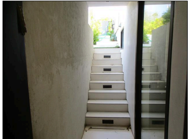
Railing Missing, Right Side Steps
