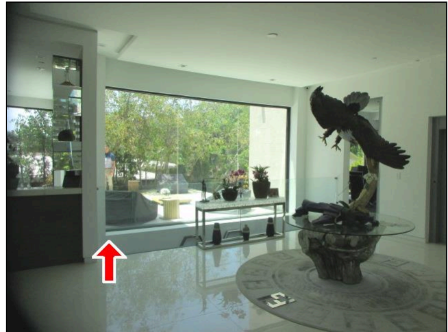
Signs Of Water Intrusion
