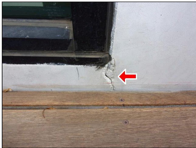
Cracked Siding, Rear Living Room Wall
