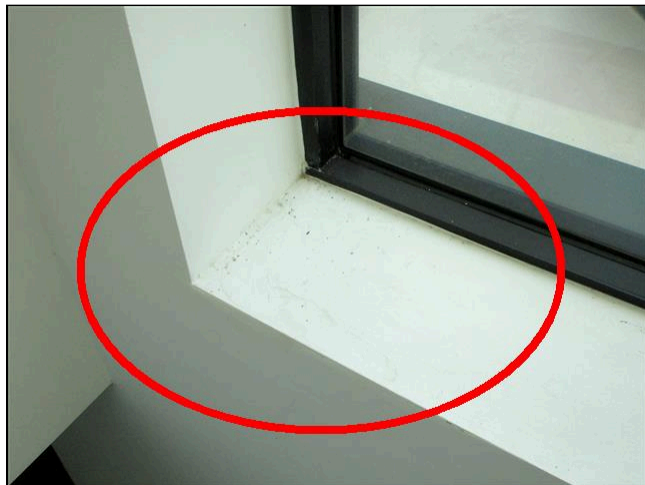
Signs Of Water Intrusion
