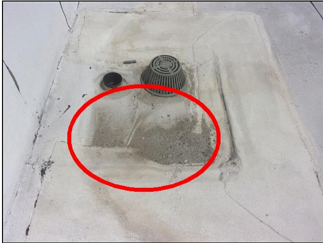
Weak Spot, Right Side Scupper
