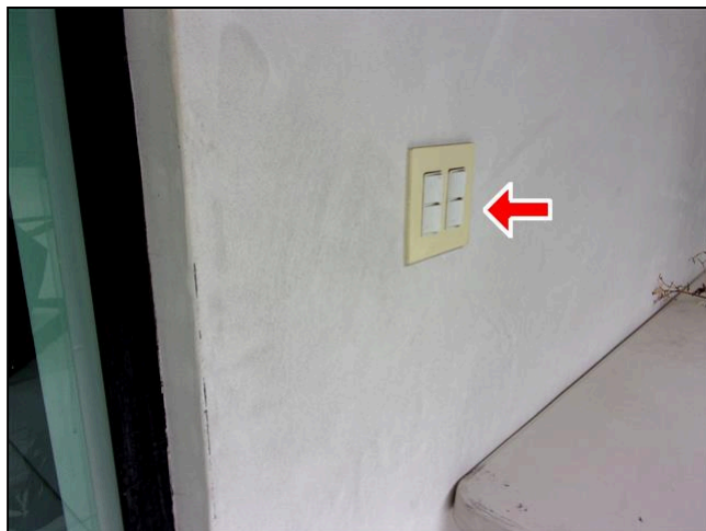
Weather Rated Cover Missing
