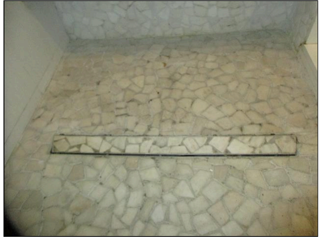
Loose Drain Cover
