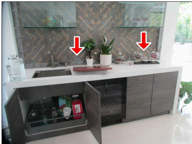
Outlets Not Operational, Kitchen
