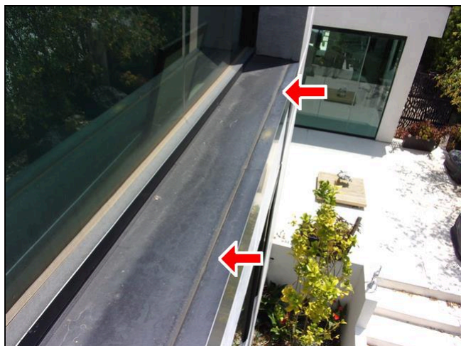
Flashing Incorrectly Sloped
