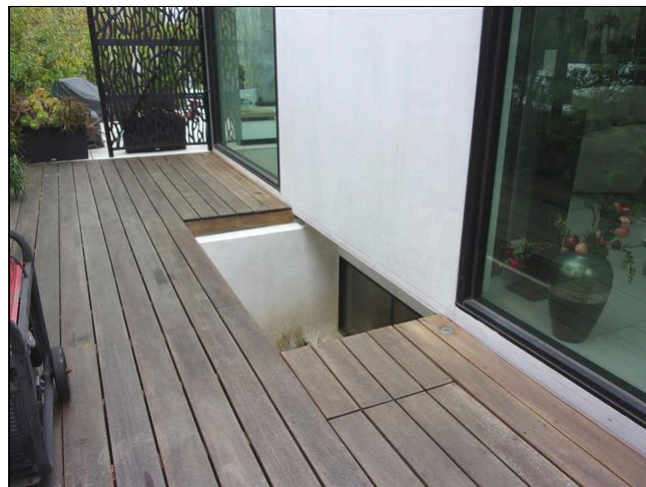
Guard Rail Missing
