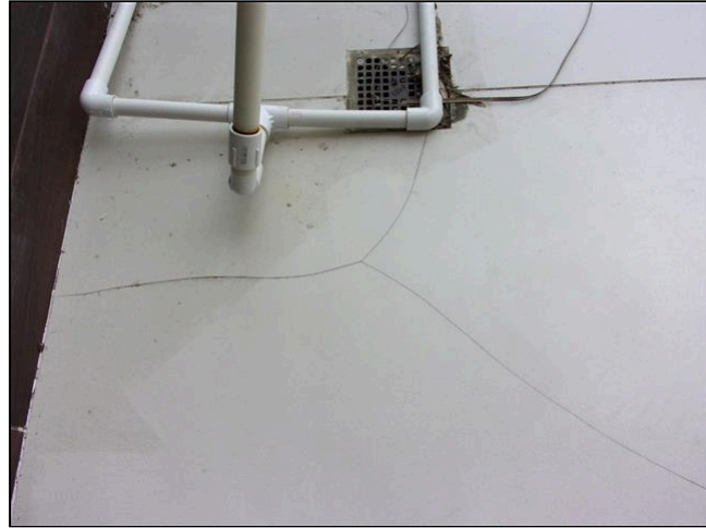
Cracked Tile Surface
