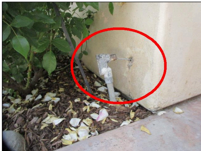
Loose Conduit, Exposed Wiring
