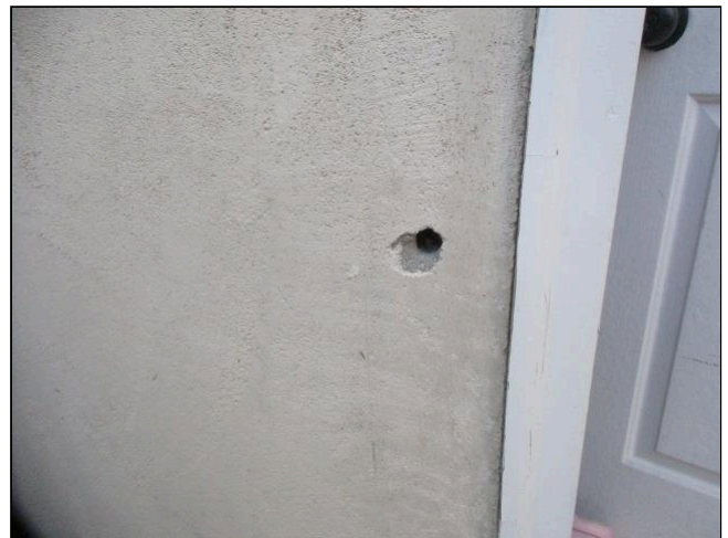
Holes In Stucco
