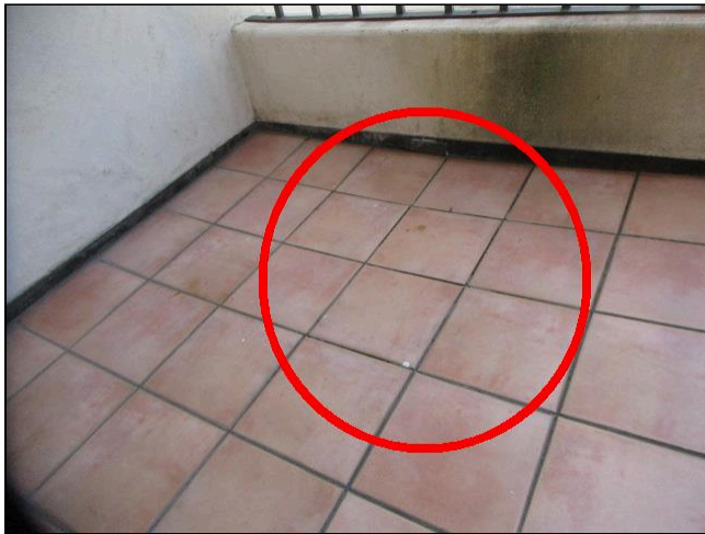
Weak Balcony Surface, Rear Guest Bedroom
