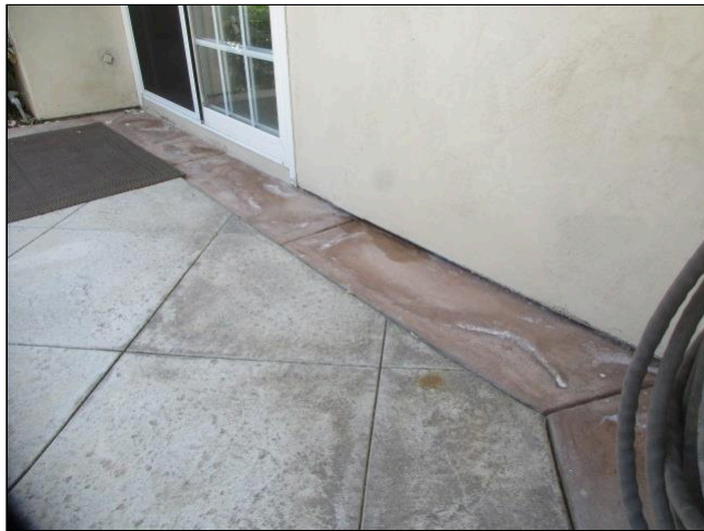
Patio Sloped Toward Home, Poor Drainage
