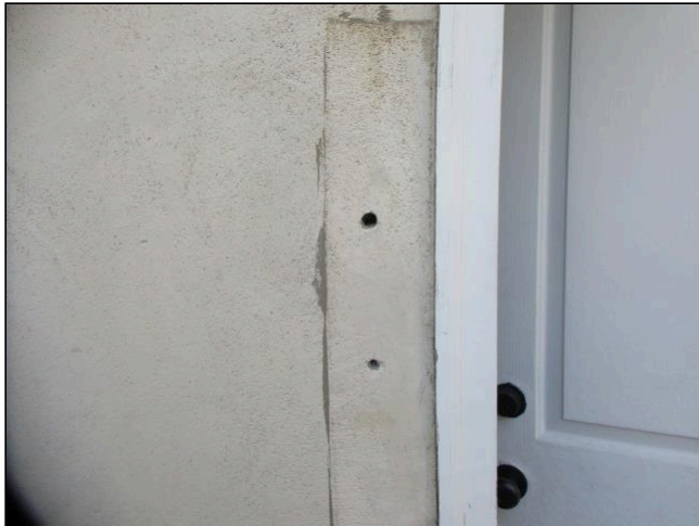
Holes In Stucco
