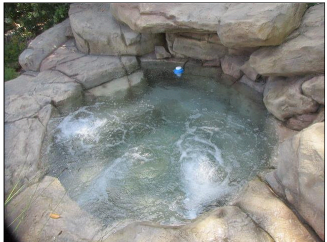
Spa Booster Pump Not Operating Properly
