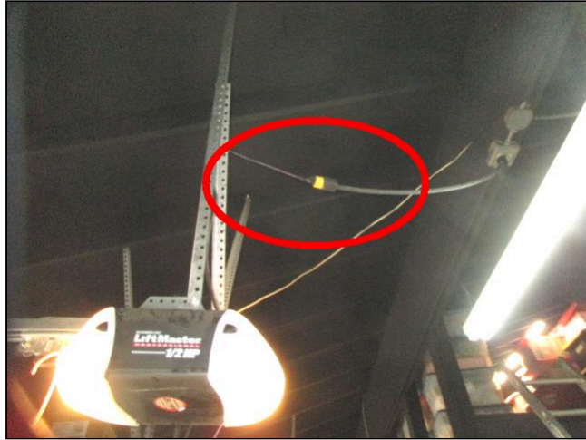
Extension Cords In Use
