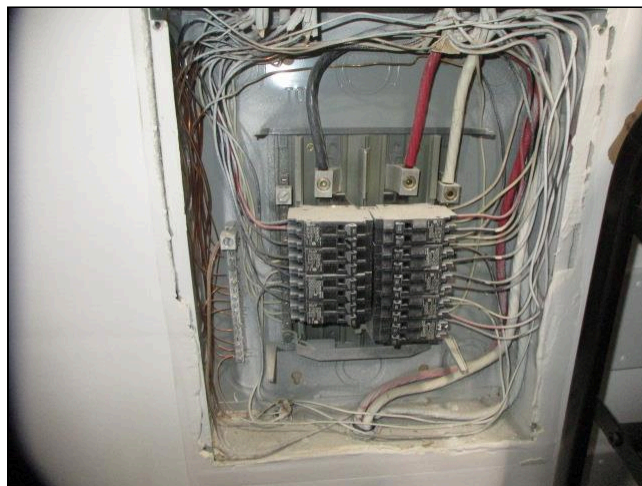
Sub Electrical Panel View, Primary Bedroom Closet
