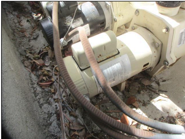
Pumps Not Bonded To Ground
