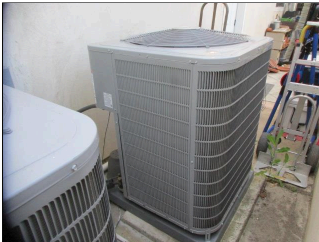
A/C Condenser View, Upstairs
