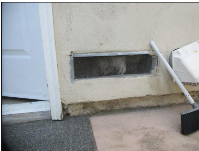
Garage Vents Blocked/Covered
