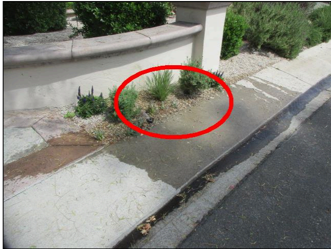
Leaking Sprinkler Piping
