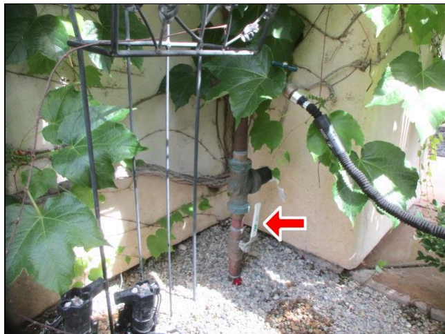
Main Water Shut Off Valve
