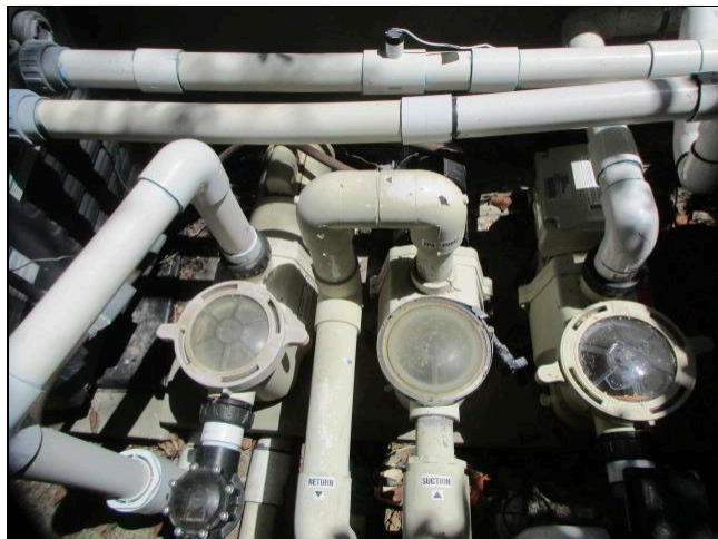
Spa Booster Pump Not Operating Properly
