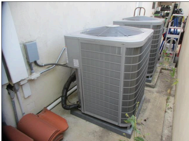
A/C Condenser View, Downstairs
