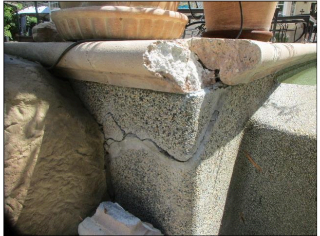
Damaged Coping, Sidewall
