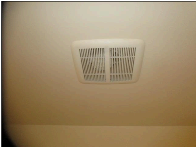
Fan Not Operational
