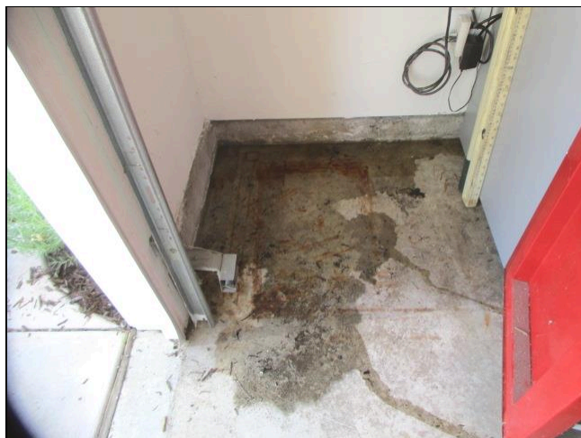
Leaking Into Garage
