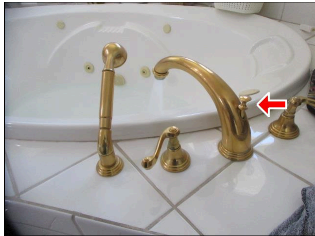
Diverter Not Operational
