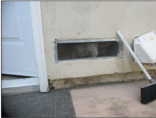
Garage Vents Blocked/Covered
