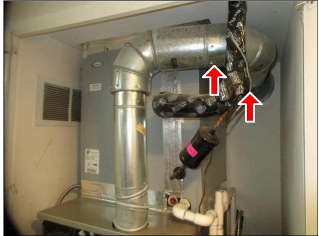
Vent Slope Improper, Downstairs Furnace
