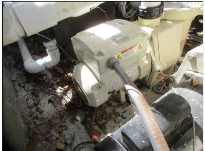
Pumps Not Bonded To Ground
