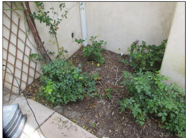
Soils Too High, Left Side
