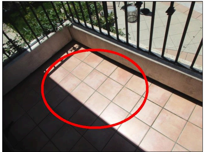
Weak Balcony Surface, Loft
