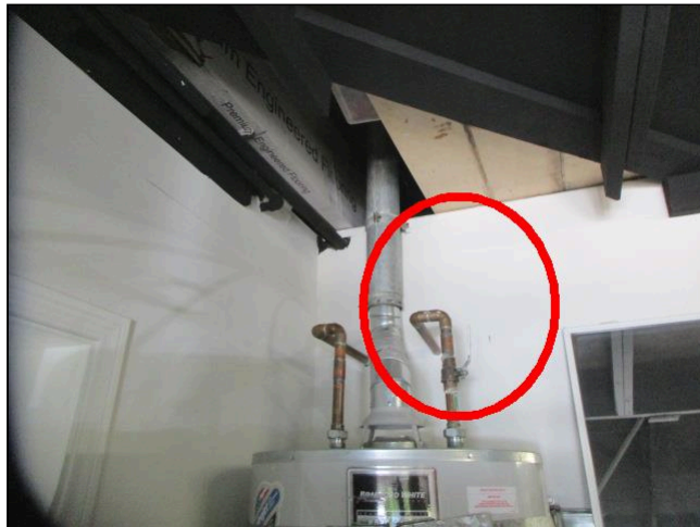
Thermal Expansion Tank Missing
