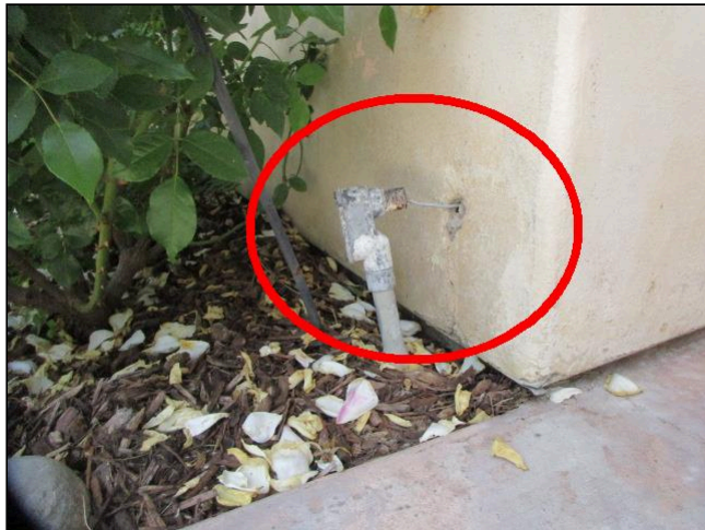
Loose Conduit, Exposed Wiring
