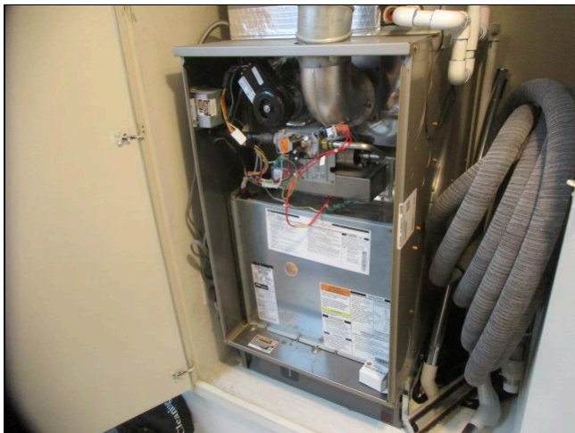
Furnace View, Downstairs System
