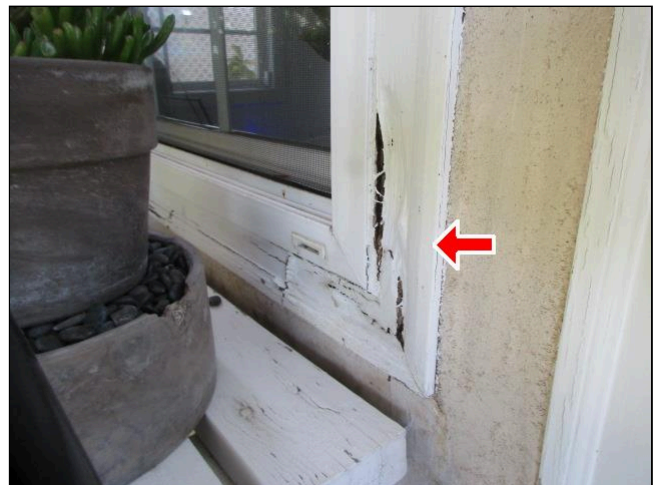
Damaged Window Banding, Family Room
