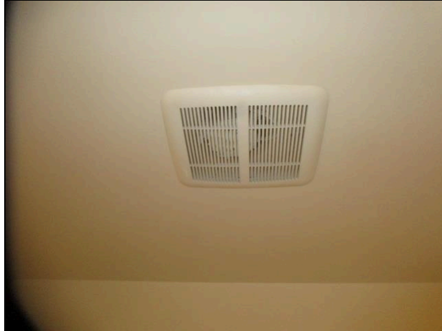
Fan Not Operational
