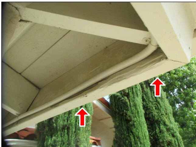
Damaged Fascia, Front
