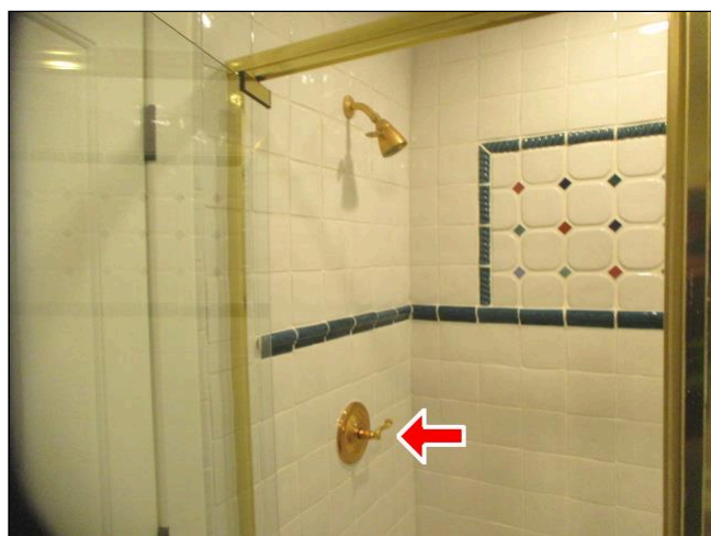
Shower Faucet Not Operational
