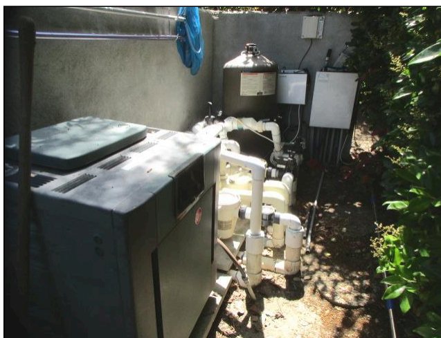
Pool/Spa Equipment View
