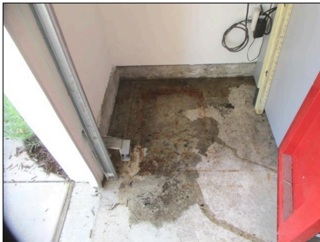
Leaking Into Garage
