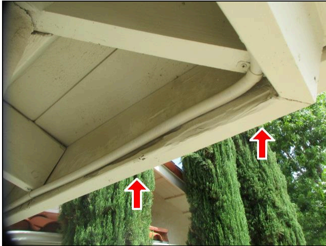
Damaged Fascia, Front
