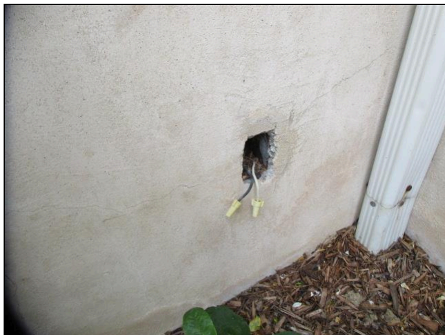
Exposed Wiring At Open Box
