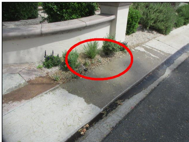
Leaking Sprinkler Piping
