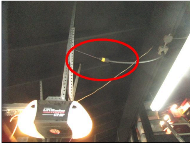
Extension Cords In Use
