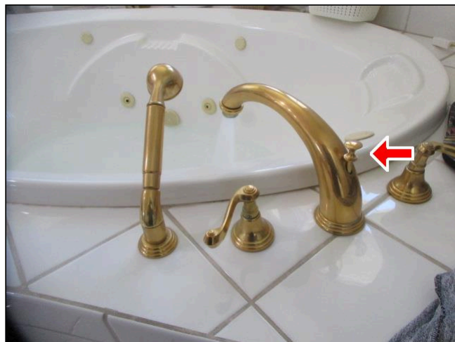
Diverter Not Operational
