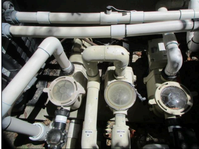
Spa Booster Pump Not Operating Properly
