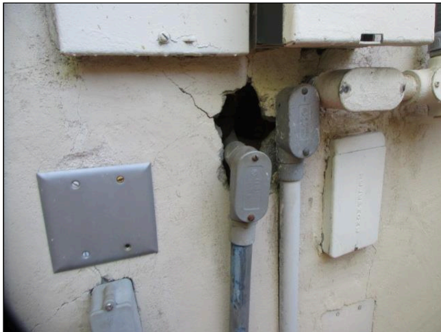
Holes In Stucco
