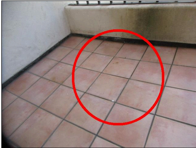
Weak Balcony Surface, Rear Guest Bedroom
