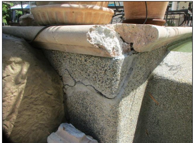
Damaged Coping, Sidewall
