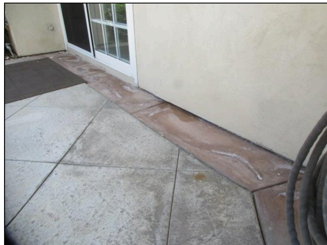
Patio Sloped Toward Home, Poor Drainage
