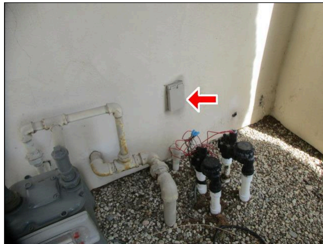
GFCI Fails To Trip
