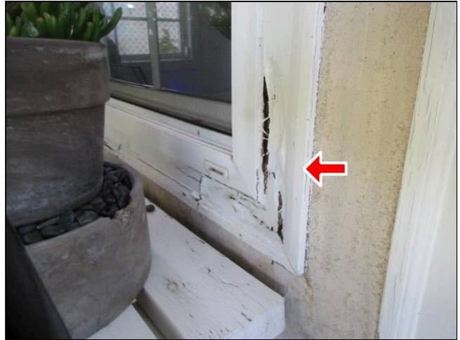
Damaged Window Banding, Family Room
