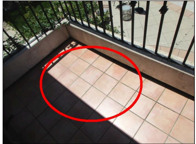
Weak Balcony Surface, Loft
