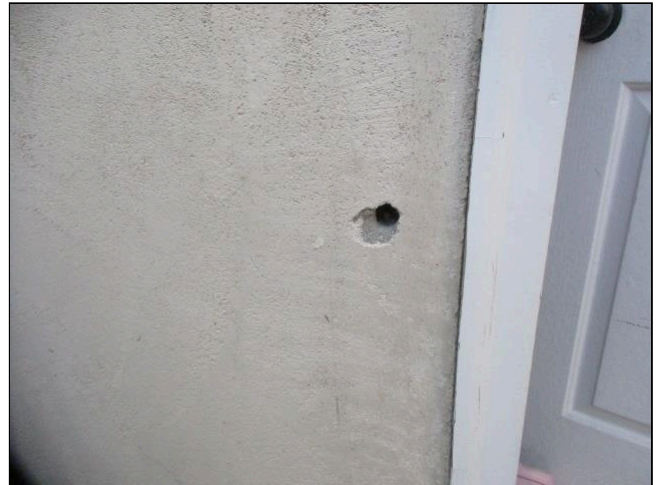
Holes In Stucco
