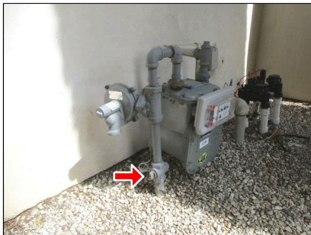
Gas Shut Off Valve
