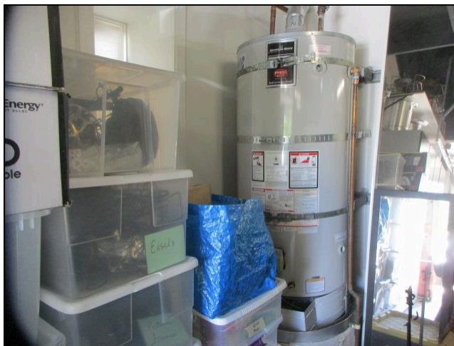
Water Heater View
