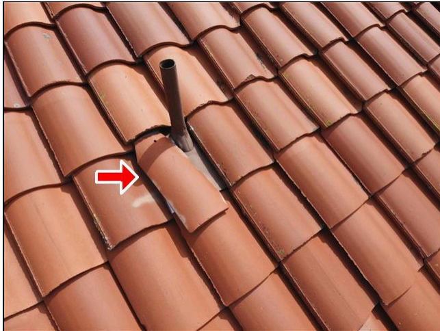
Loose Tile, Left Side
