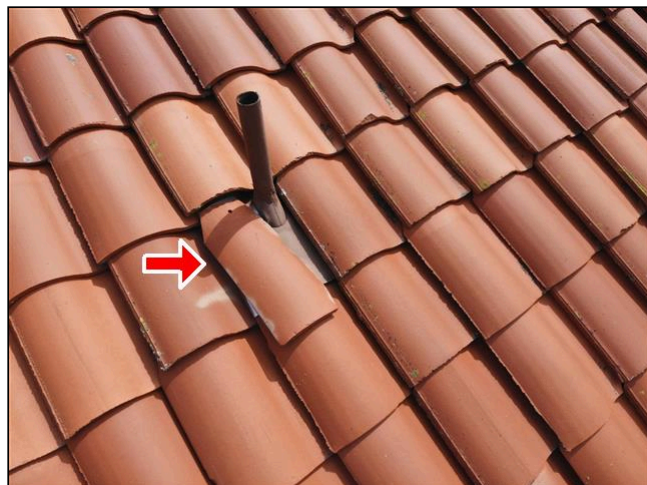
Loose Tile, Left Side
