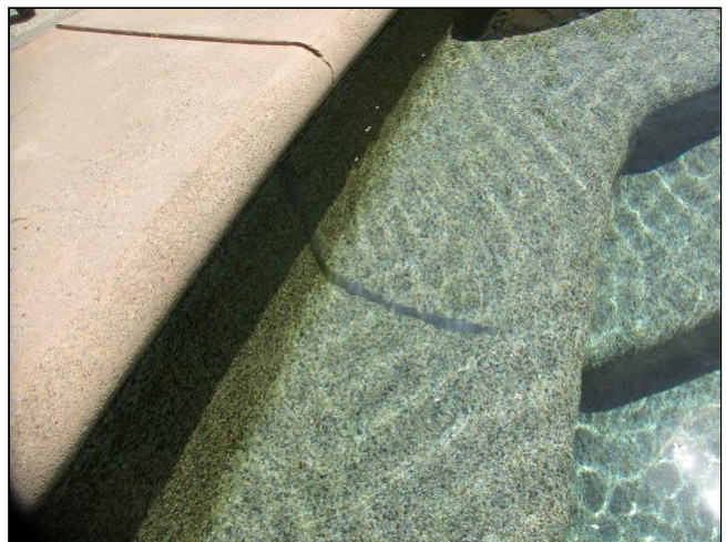
Previous Repairs, Pool Steps
