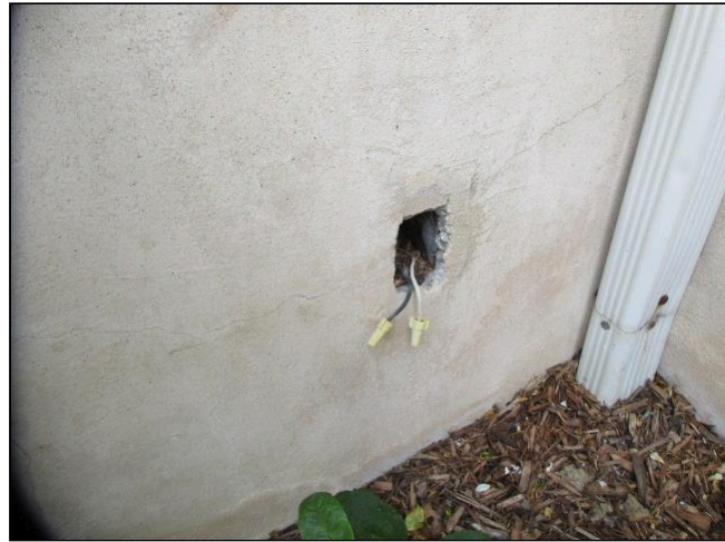
Exposed Wiring At Open Box
